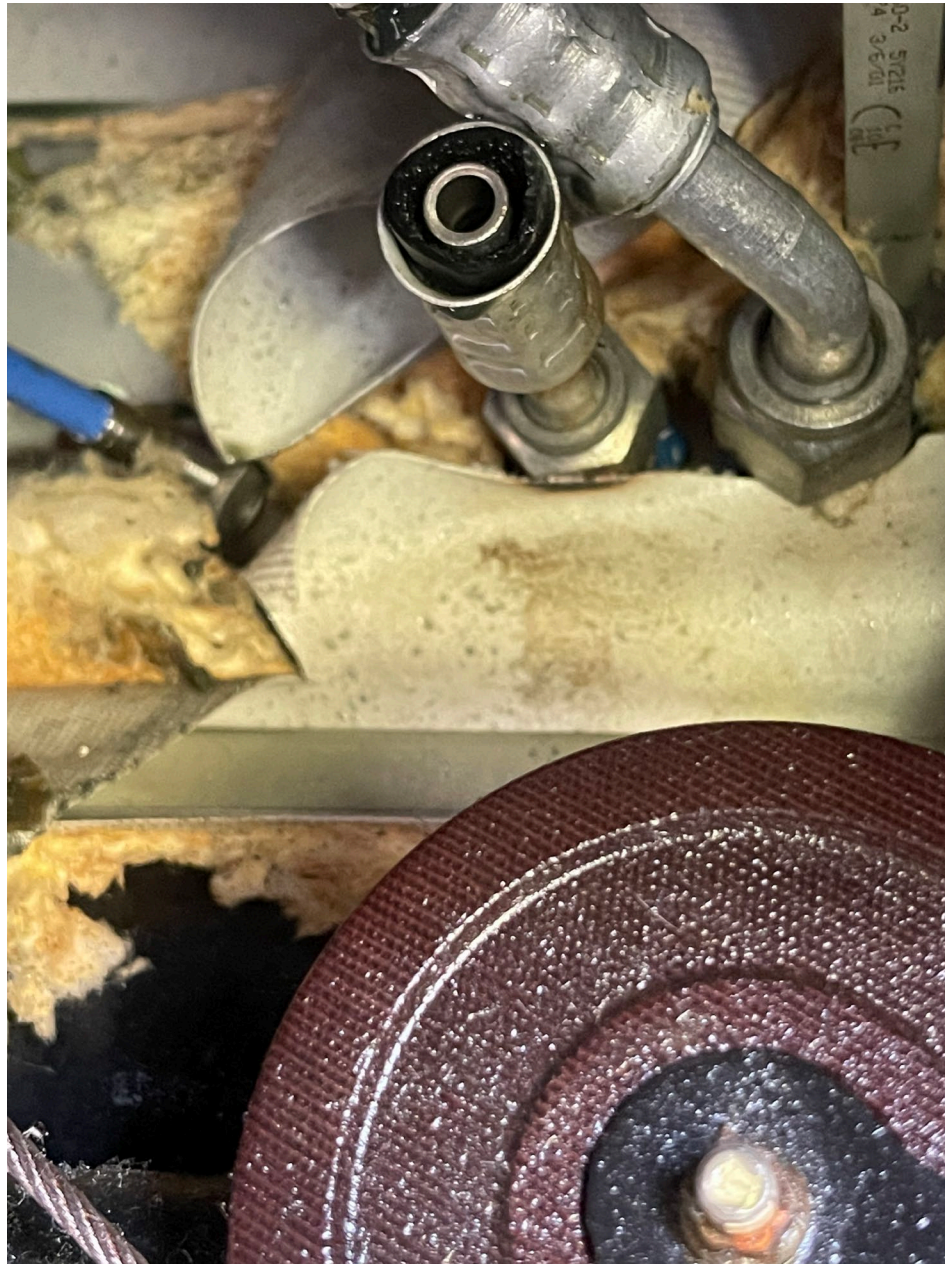
Photo 6 – Close up view of the rubber air conditioning hose that failed at the metal crimp connection (courtesy of the Federal Aviation Administration).
