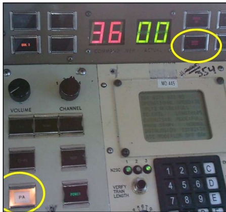
Door Open present--now make ADA announcement
