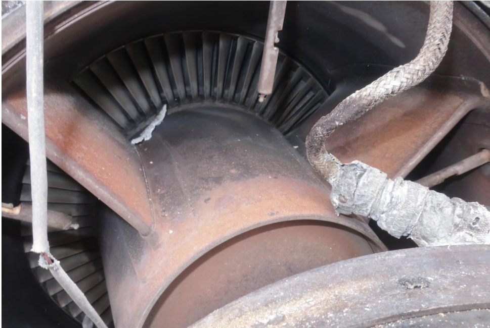
Figure 10. Second stage power turbine section showing no missing, ruptured, or burned blades.
