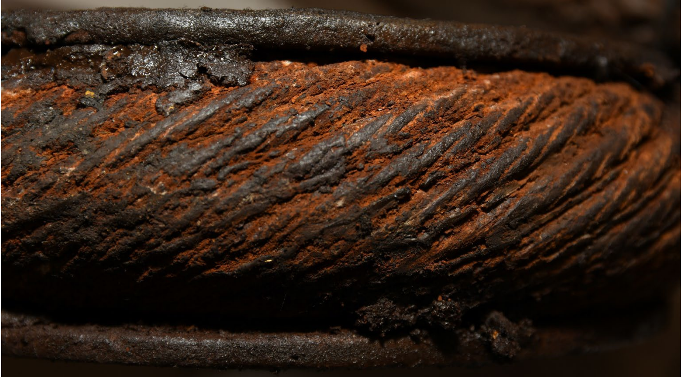
Figure 6 Image showing the rough surface and heavy corrosion product buildup at the eye on Specimen 1 (74-1). (Severity Rating 60%)
