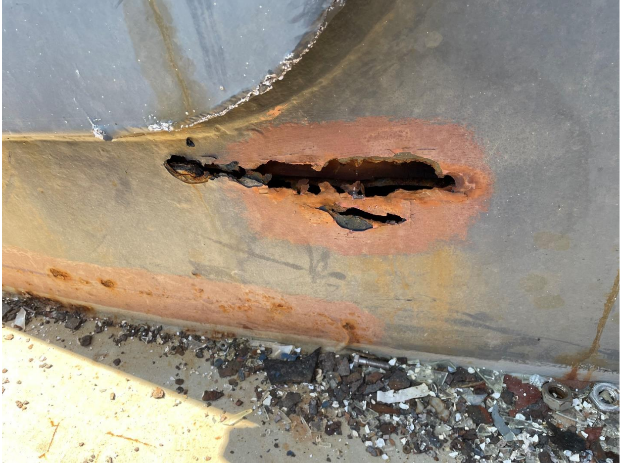
Wastage, port deckhouse
