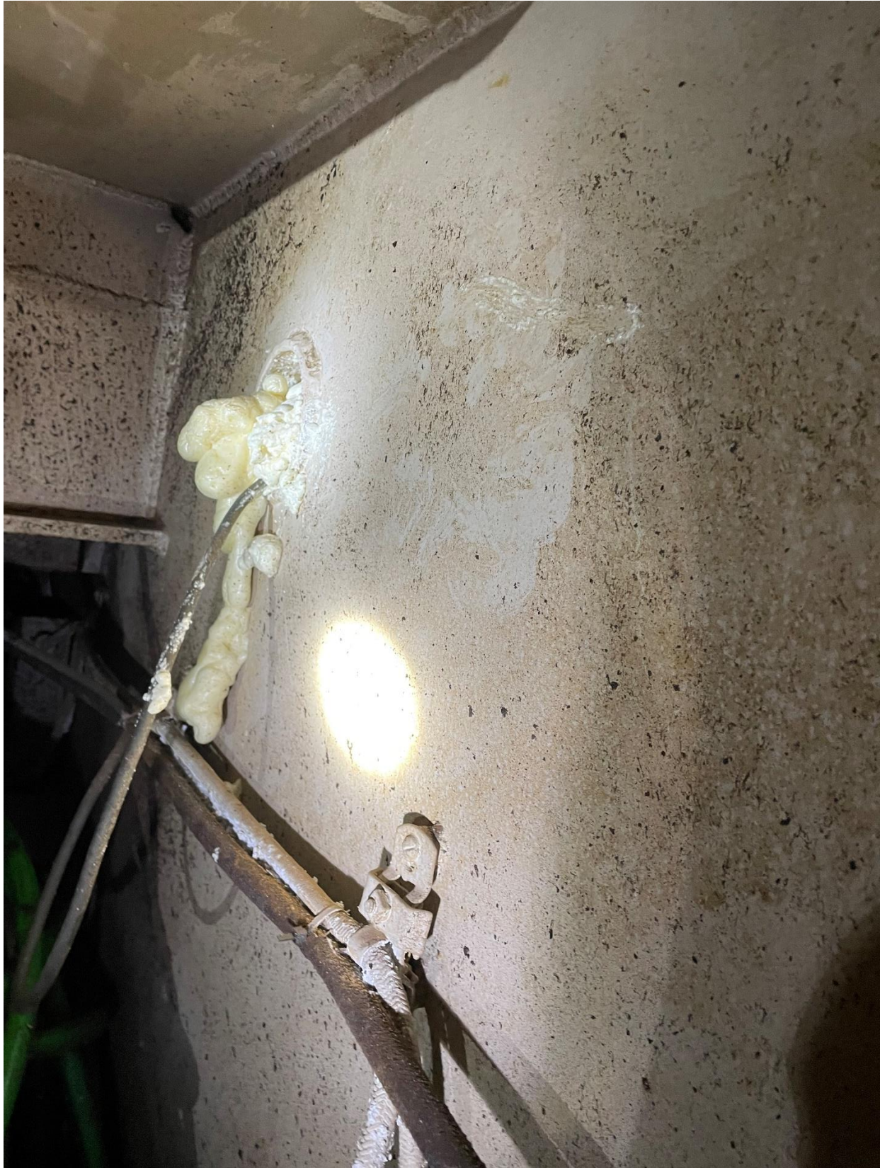
Wire run opening, aft engine room bulkhead (foam added during salvage post-sinking)
