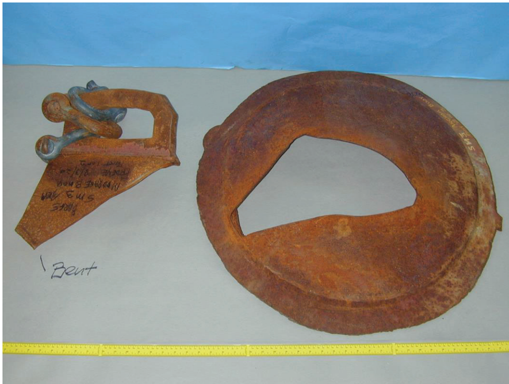
Fig. 1: Overall view of the submitted failed section that had reportedly been removed from the buoy (see Attachment 2-3) utilized in the moorage arrangement of barge SM3.
