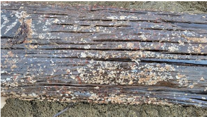
164. Pile No 10 – fender pile with surface checking
