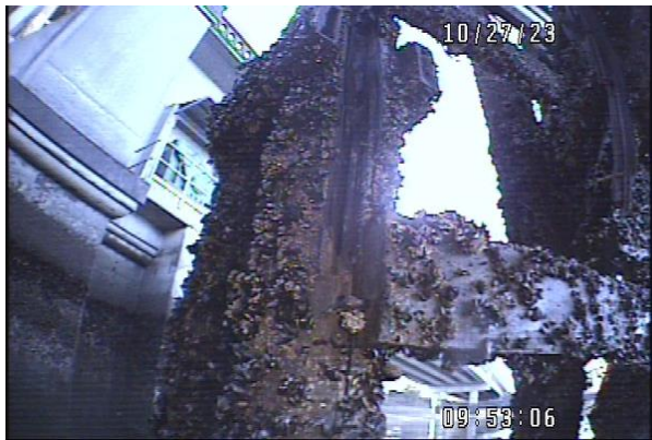
63. No. 6 pile – rotten above waterline
