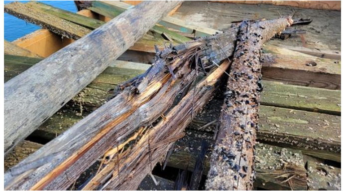
209. No 4 batter pile – checking over surface area and core deteriorated
