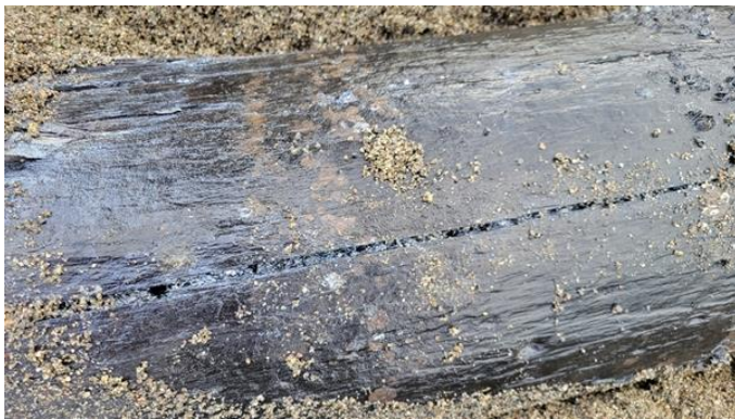
168. No 12 fender pile – broken off below mudline and with surface checking
