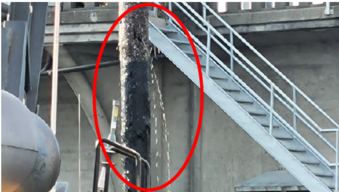
242. No 26 fender pile – leaking water due to hollow sections in core
