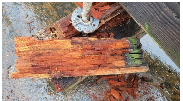
121. Catwalk timber soft and powdery
