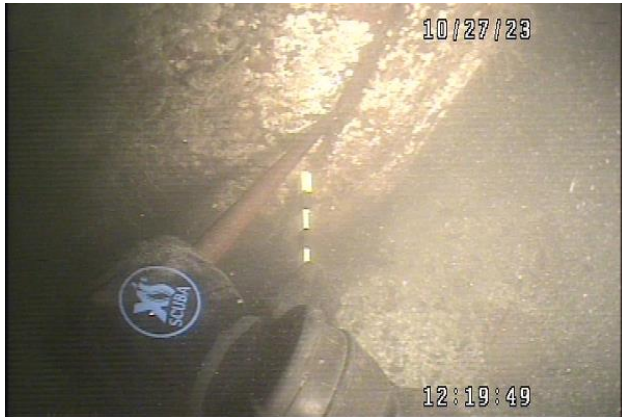
100. Fender cluster 4 – S pile – core rot measured at 11” at base with rot extending up to half of pile height
