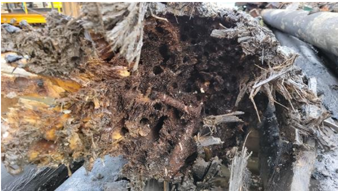
224. Heavily deteriorated core and worm tracks
