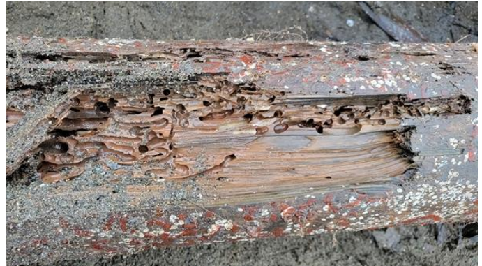
199. No 2 pile cluster – core degradation and worm tracks
