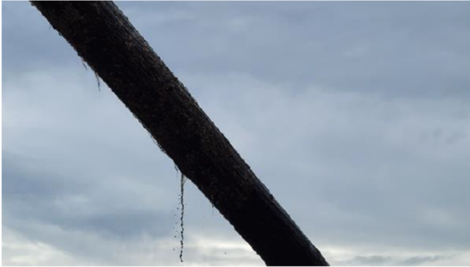
232. No 3 pile 4 th cluster – water leaking during lifting due to hollowed core
