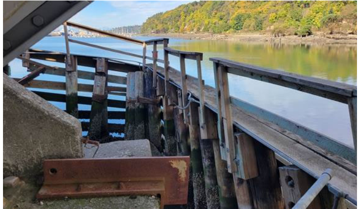
24. Damaged sheer wall
