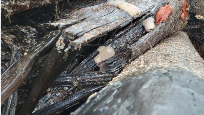
188. No 3 pile cluster – broken and with hollow cores
