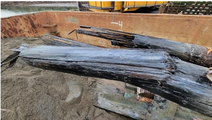
150. Pile No 21 – broken off below mudline
