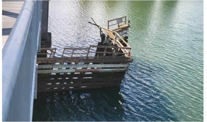
20. Damaged sheer wall
