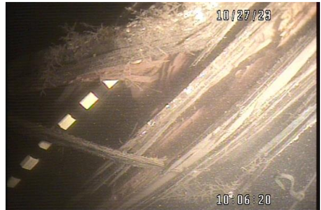
66. No. 8 batter pile – core rotten
