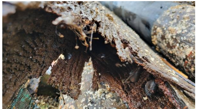
225. Horizontal support - core deterioration
