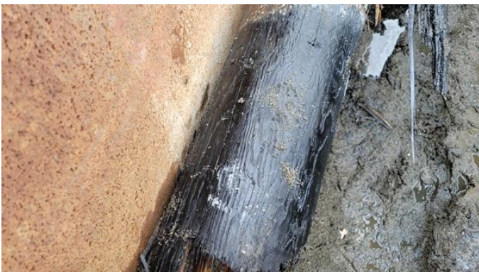
180. No 17 fender pile – surface checking and pressure flowering
