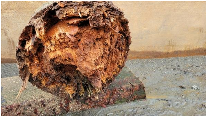
128. Top of Pile No 27 – visually poor condition, core rotten, very powdery
