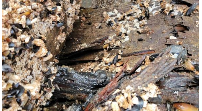
163. Pile No 9 – fender pile with core degradation
