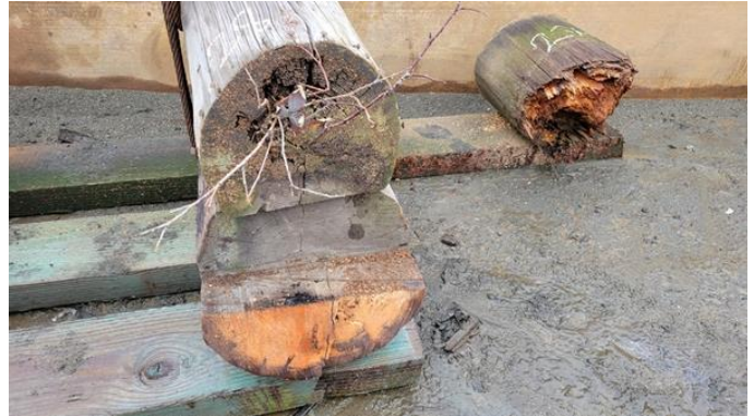
127. Top of Pile No 28 – core deterioration visually observed
