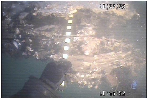
73. No. 10 pile – horizontal cap timber – heavy rot
