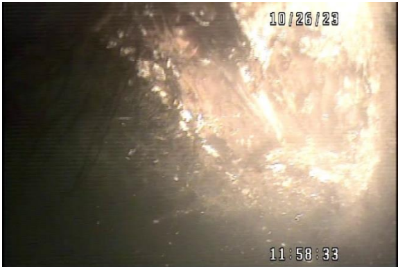
43. No 8 batter pile – bottom section loss
