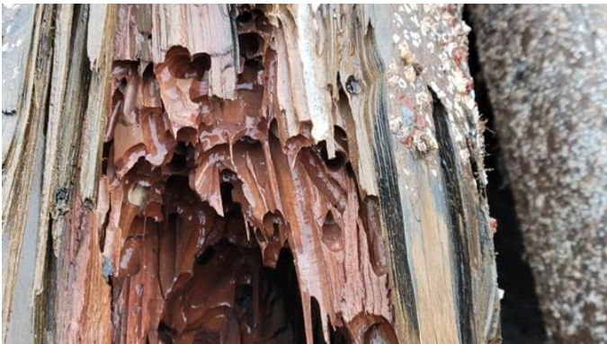
194. No 2 pile cluster – core degradation and worm tracks
