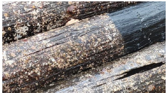
235. No 31 fender pile – pressure flowering at mudline interface
