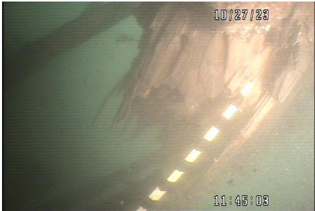
91. Fender cluster 3 SE pile – broken with heavy rot
