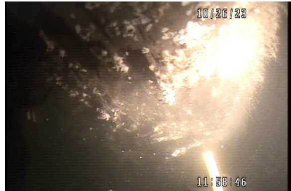
44. No 8 batter pile – worm tracks and rot
