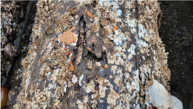
172. No 14 fender pile – surface degraded and with worm tracks
