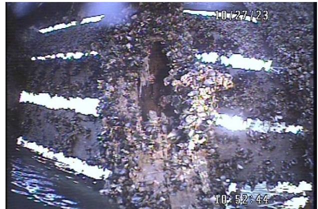
76. No. 10 pile – heavy core rot sighted above waterline
