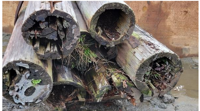
131. Top of No 4 cluster – extensive core deterioration observed
