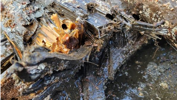
212. No 1 cluster pile – core degradation and extensive worm tracks
