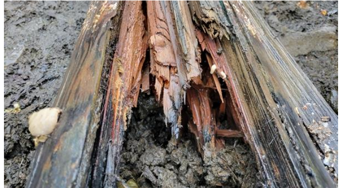
149. Pile No 20 batter pile – broken off at mudline – wastage of core and heavy worm tracks noted
