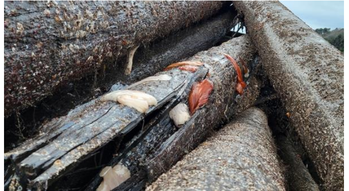
189. No 3 pile cluster – broken and with hollow cores
