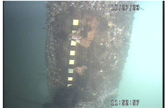
96. No. 24 pile – north and south horizontal supports missing
