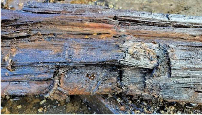
204. Pile cluster No 1 top – timber deteriorated
