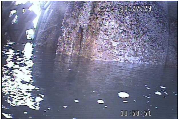
77. No. 12 pile – pier connected board rot
