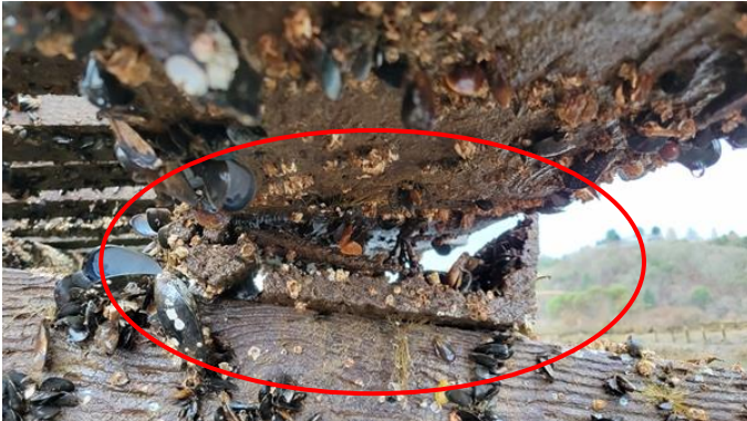
162. Pile No 9 – fender pile with core degradation
