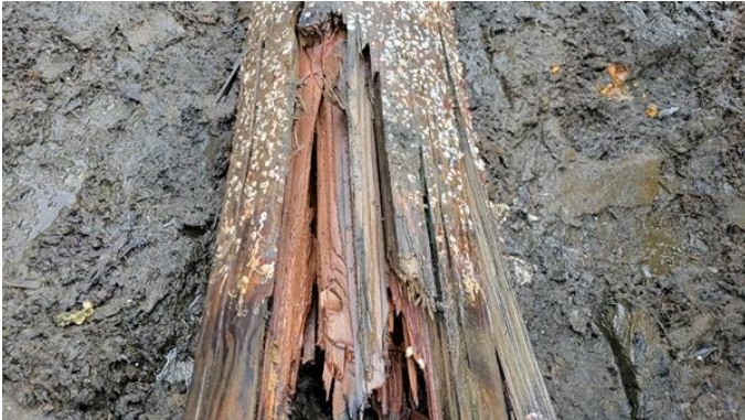
148. Pile No 20 batter pile – broken off at mudline – wastage of core and heavy worm tracks noted
