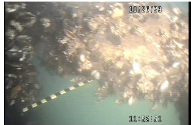
42. No 6 pile – heavy marine growth
