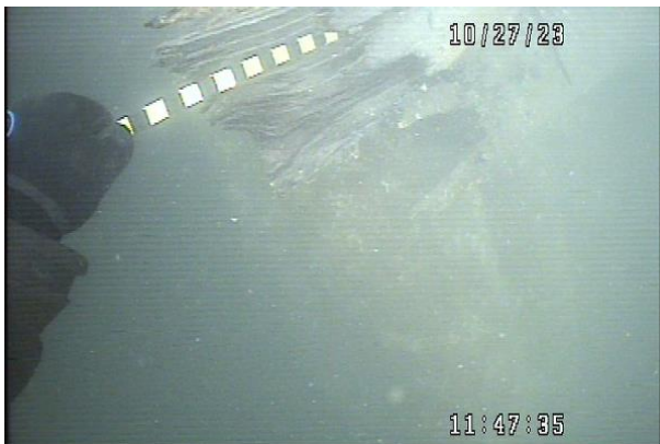
93. Fender cluster 3 – connecting fenders rotten and broken off
