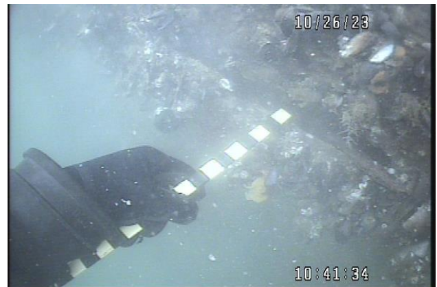
26. No 1 Batten with end rot and loss
