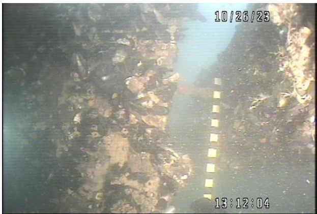
49. No 24 pile – gap between pile cap and timber
