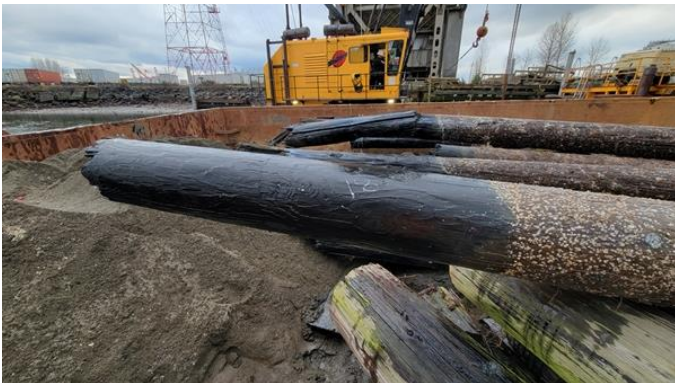
136. Pile No 18 – broken off below mudline
