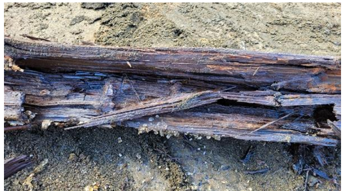
207. Pile cluster No 1 top – timber deteriorated
