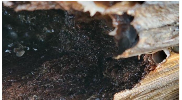
175. No 14 fender pile – hollow with no core strength
