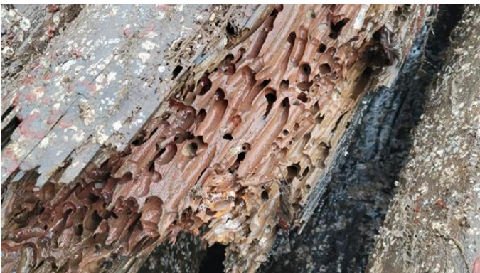
196. No 2 pile cluster – core degradation and worm tracks
