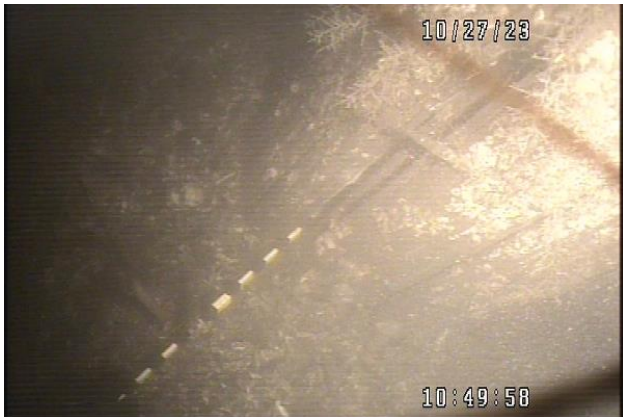
75. No. 10 pile – heavy checking below waterline – possible internal core rot
