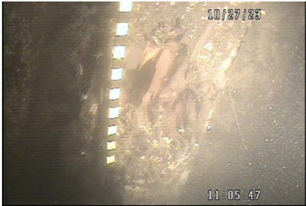
81. No. 15 pile – broken with over 90% core loss at 22’
