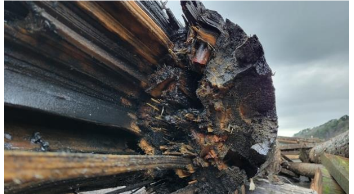
153. Pile No 22 – broken off at mudline – wastage of core observed
