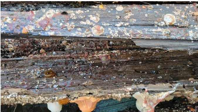
174. No 14 fender pile – hollow with no core strength
