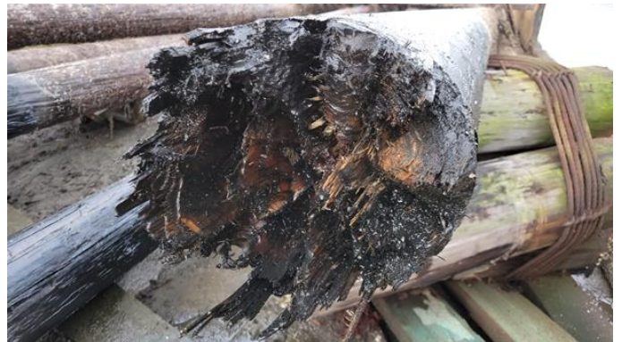
137. Pile No 18 – lower section – interior core wasted and soft to touch.
