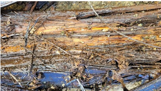
206. Pile cluster No 1 top – timber deteriorated
