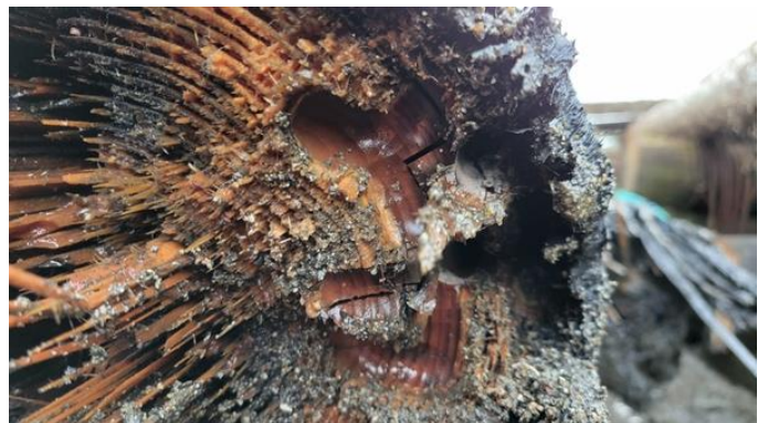
181. No 17 fender pile – core degradation and worm tracks observed
