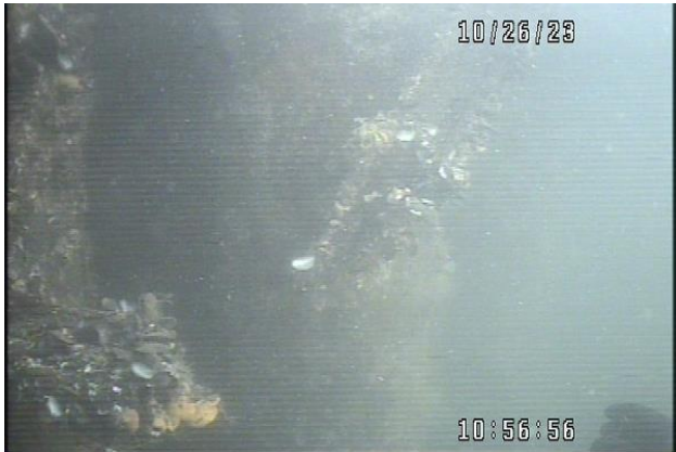
27. No 1 BC Interface - section missing
