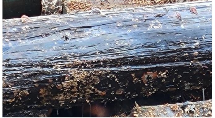
237. No 30 fender pile – section loss due to borers.
