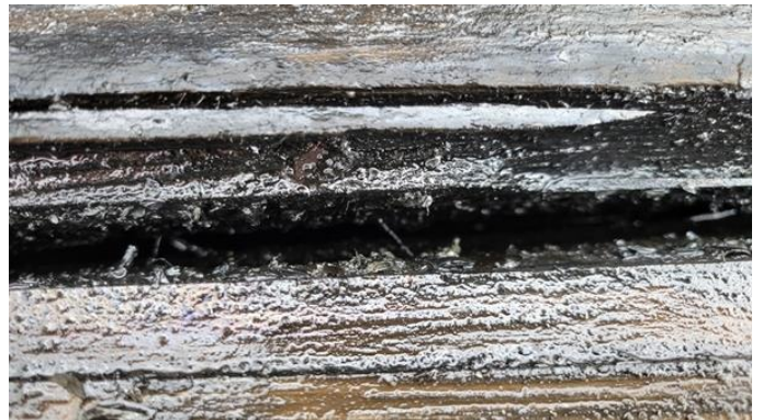
143. Pile No 19 – cracks observed over length of pile
