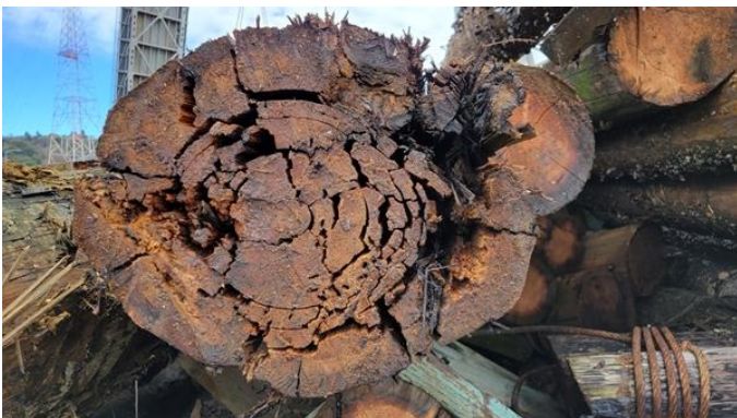
220. Pile Nos 1-6 – general deterioration
