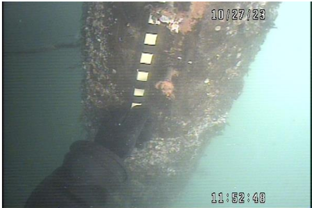
95. No. 24 pile – north and south horizontal supports missing
