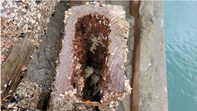
140. Pile No 18 lower horizontal support – extensive core wastage noted.
