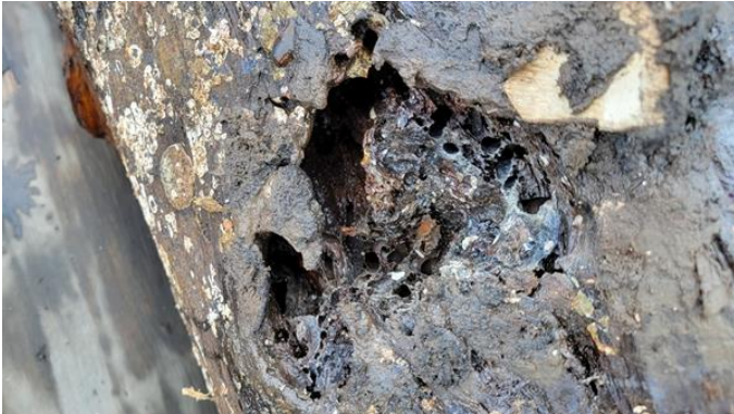
222. Heavily deteriorated core and worm tracks
