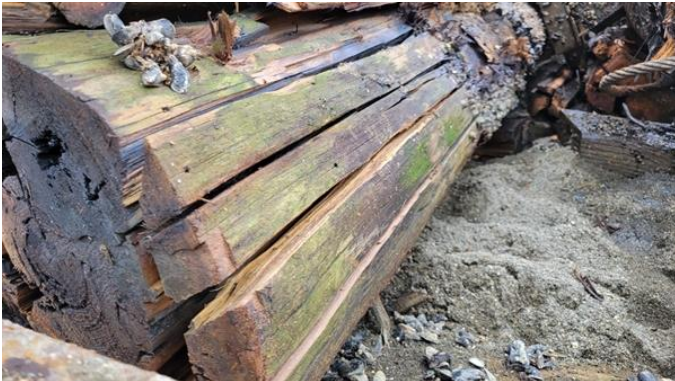
218. Pile Nos 1-6 – general deterioration
