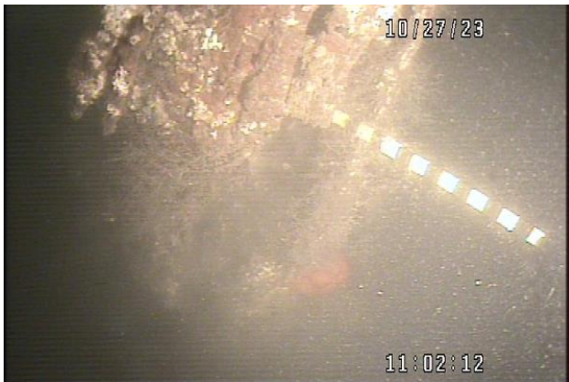
79. No. 14 pile – rot at 15' down with 90% section loss
