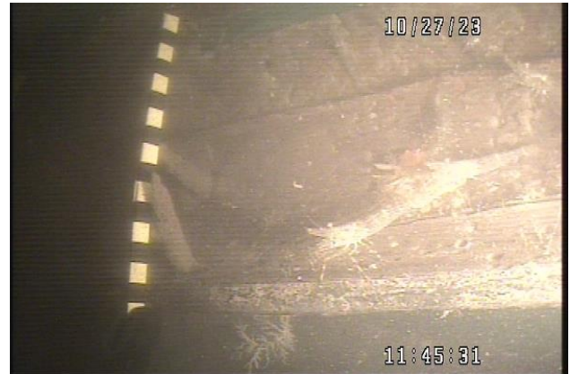
92. Fender cluster 3 SW pile – severed above mudline and core hollowed out.
