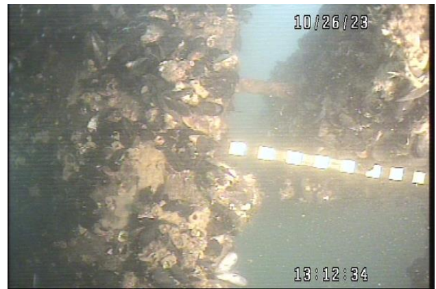
50. No 24 pile – gap between pile cap and timber
