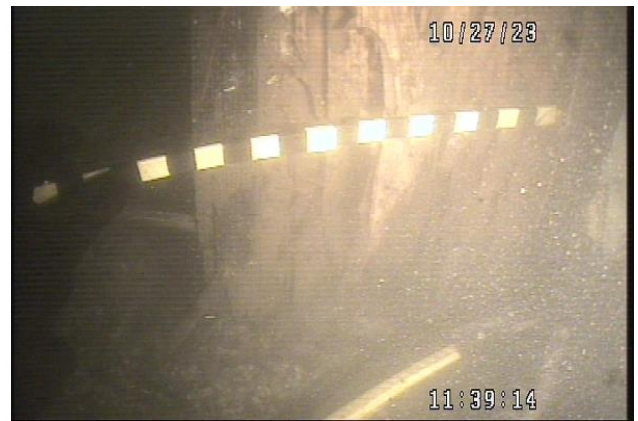
88. Fender Cluster 3 SE pile – broken with heavy rot
