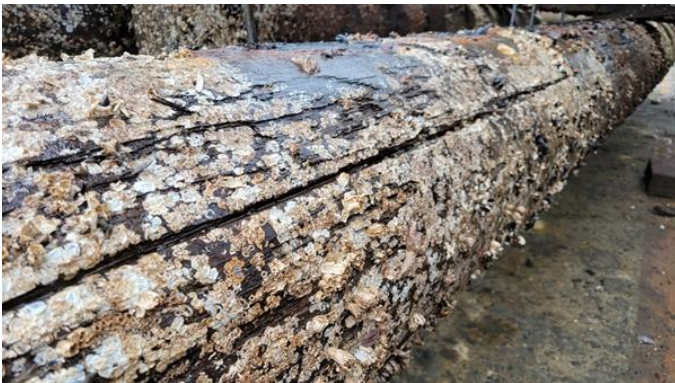
142. Pile No 19 – cracks observed over length of pile
