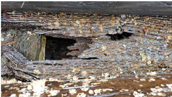
226. No 28 batter pile – core hollowed out at mudline interface
