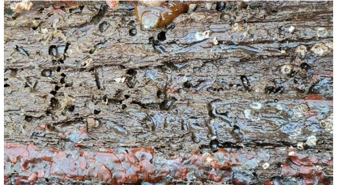
173. No 14 fender pile – surface degraded and with worm tracks
