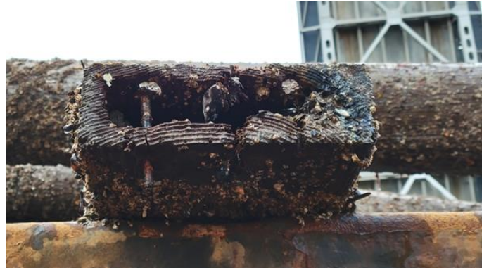
193. No 2 pile cluster – fender board with internal core degradation
