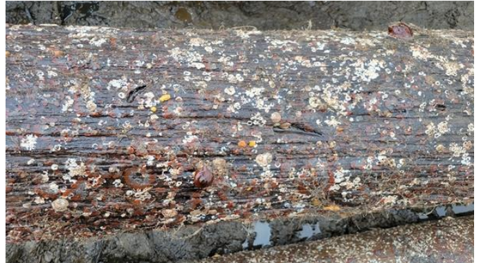
145. Pile No. 20 – worm tracks observed
