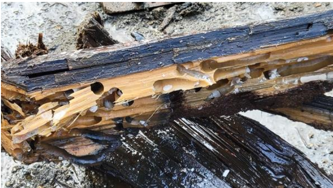
214. No 1 cluster pile – core degradation and extensive worm tracks
