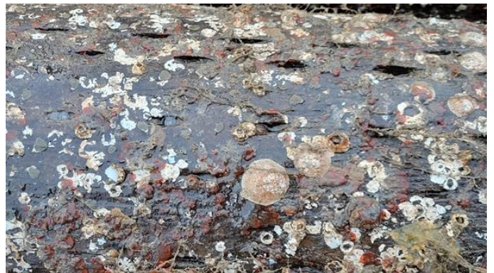
197. No 2 pile cluster – surface checks due to internal core rot
