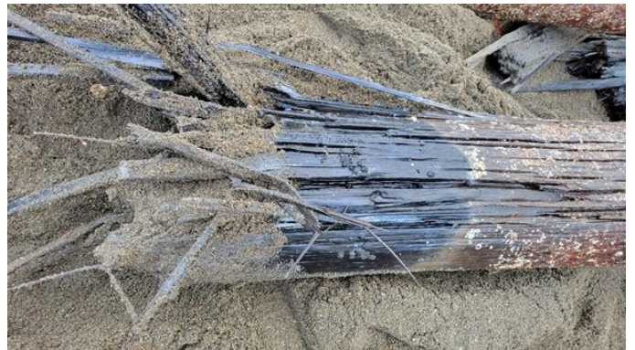
165. Pile No 10 – fender pile with surface checking and core rot
