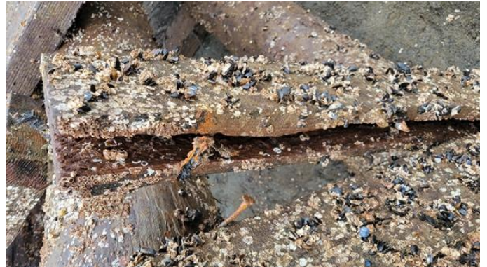
141. Pile No 18 lower horizontal support – extensive core wastage noted.
