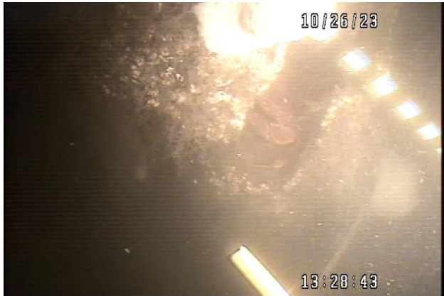
55. No 27 batter pile – fractured at mudline
