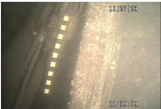
89. Fender Cluster 3 SE pile – broken with heavy rot
