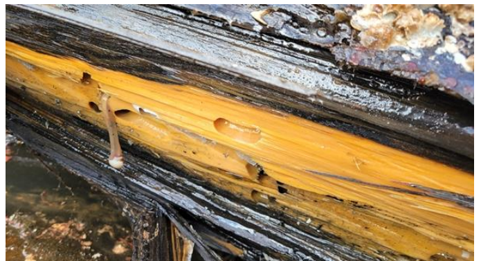
211. No 1 cluster pile – core degradation and extensive worm tracks
