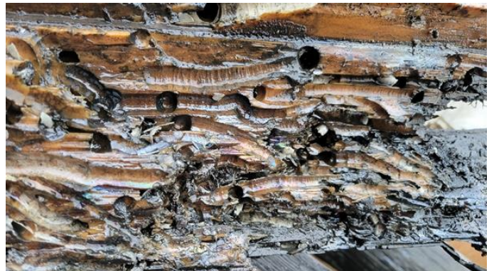
151. Pile No 21 – extensive wastage of core with worm tracks noted
