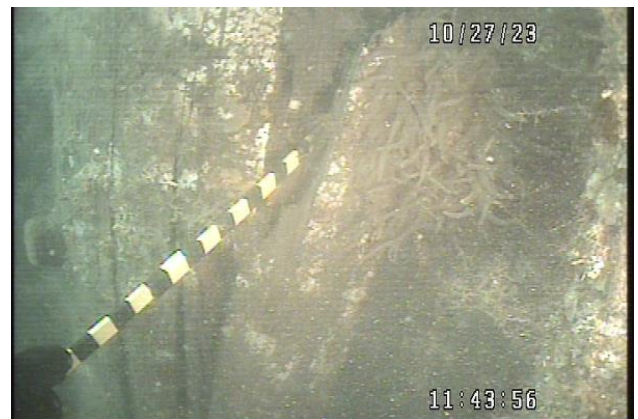
90. Fender Cluster 3 SW pile – wood sighted as rotten
