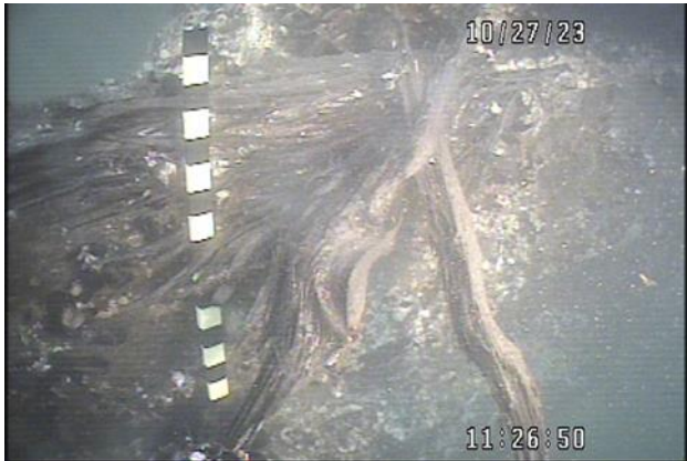
59. Batten 3 D-E section – apparent impact damage.
