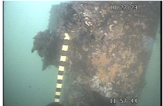
60. Batters at section G to F displaying heavy end rot. South section of G missing.
