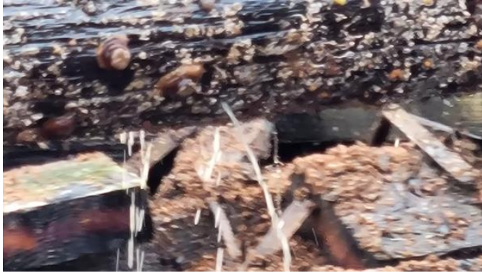
236. No 30 fender pile – leaking water from hollowed core
