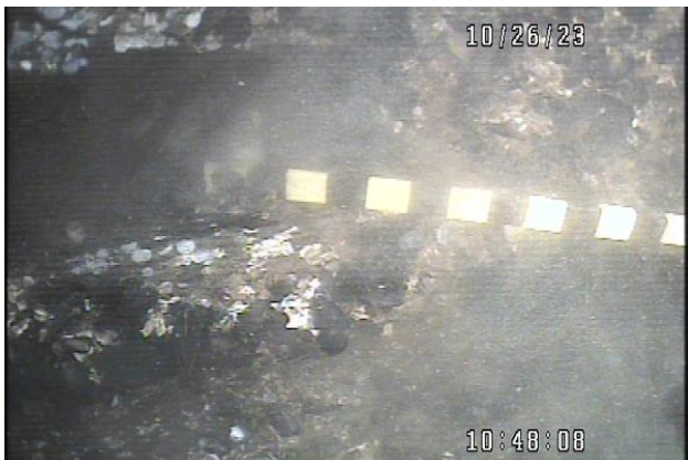
33. No 2 Batten B end with end rot
