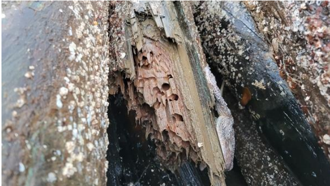
198. No 2 pile cluster – core degradation and worm tracks
