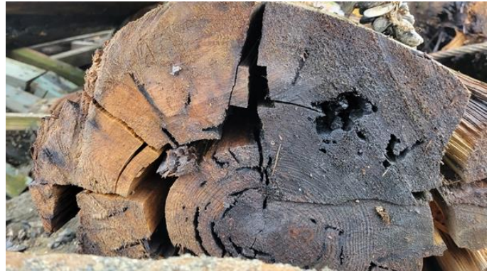
219. Pile Nos 1-6 – general deterioration
