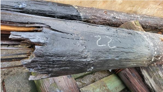
152. Pile No 22 – broken off at mudline – wastage of core observed
