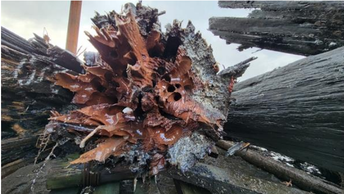
176. No 15 fender pile – broken with heavy core loss and worm tracks
