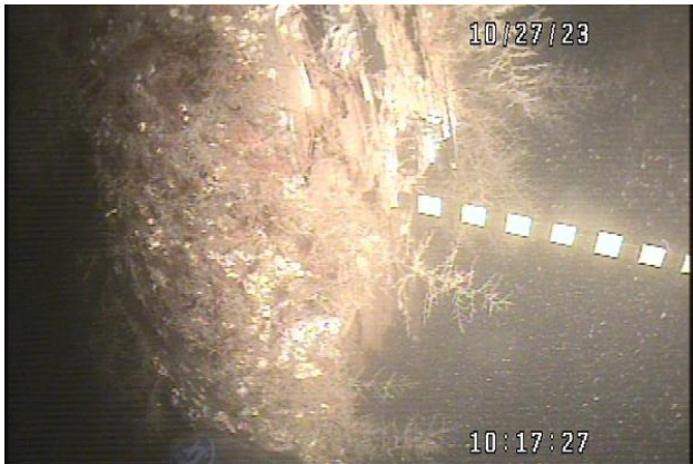
71. No. 2 pile cluster – SE pile – rot with worm tracks
