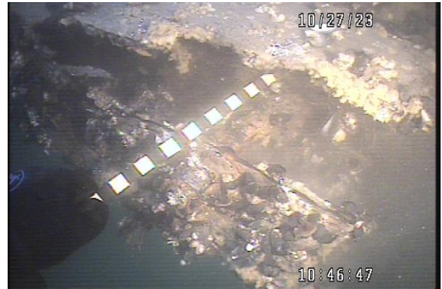
74. No. 10 pile – securing hardware degraded and heavy core rot
