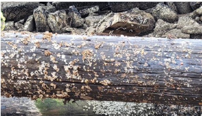
234. No 31 fender pile – light surface checking
