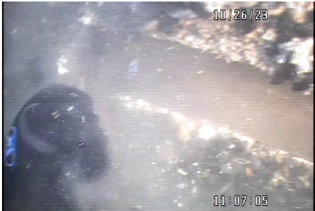
31. No 1 D batten complete core loss
