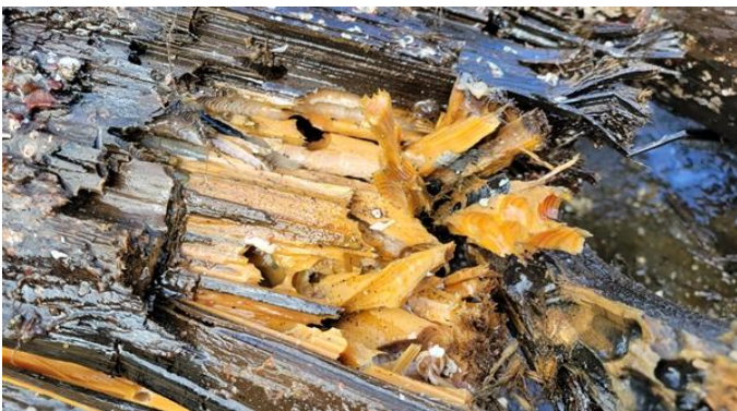
210. No 1 cluster pile – core degradation and extensive worm tracks
