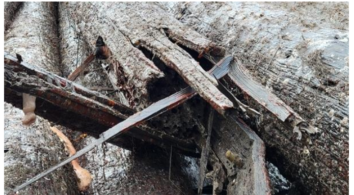
185. No 3 pile cluster – heavy degradation
