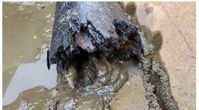
139. Pile No 18 batter pile – lower section – interior core heavily wasted
