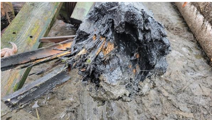
156. Pile No 22 batter pile – wastage of core
