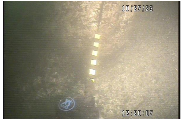
101. Fender cluster 4 – S pile – core rot measured at 11” at base with rot extending up to half of pile height
