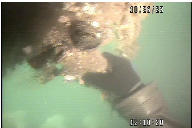
47. No 17 pile – lower section missing
