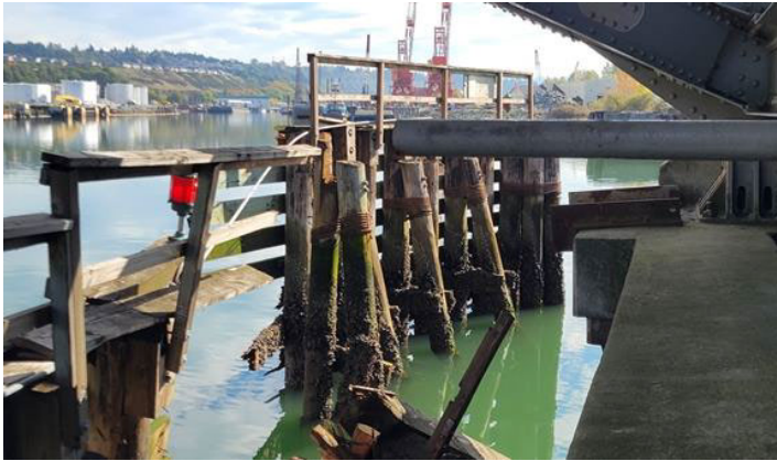
21. Damaged sheer wall
