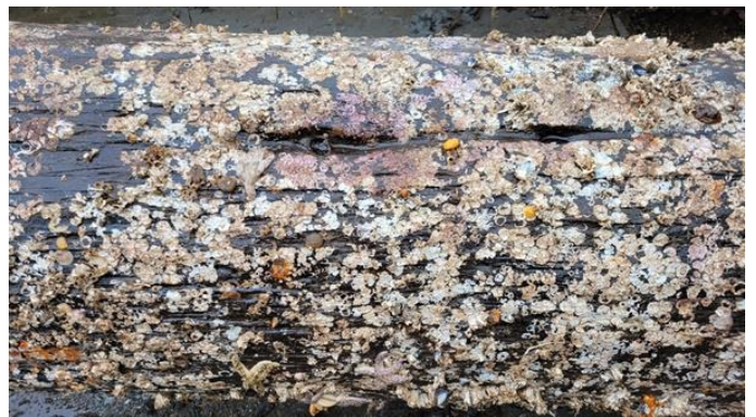
157. Pile No 22 batter pile – wastage of core and surface checking
