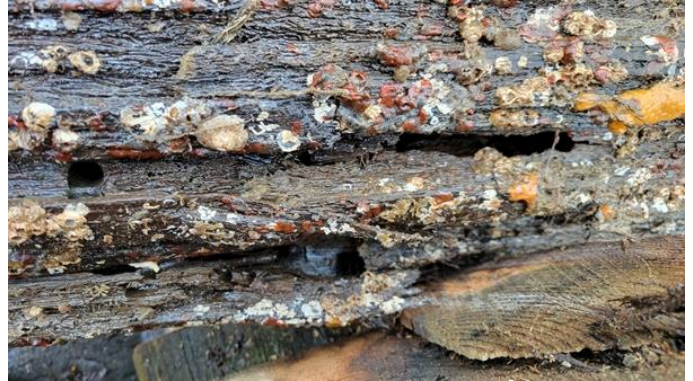
159. Pile No 23 – core loss due to borers
