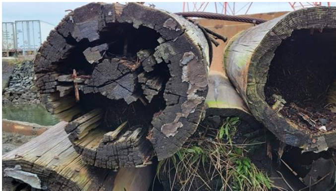
132. Top of No 4 cluster – extensive core deterioration observed
