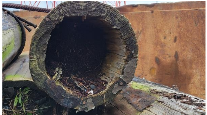
133. Top of No 4 cluster – extensive core deterioration observed
