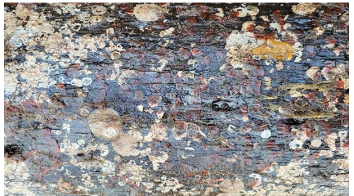
169. No 12 fender pile – core degradation due to borer worms
