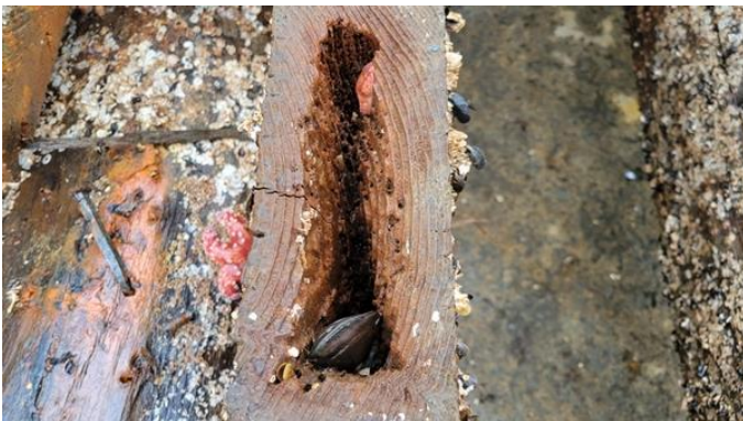
146. Pile No 20 horizontal support with core loss.
