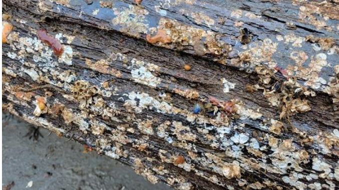
158. Pile No 23 – core loss due to borers
