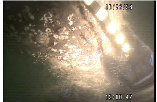
46. No 16 batter pile – worm tracks and rot
