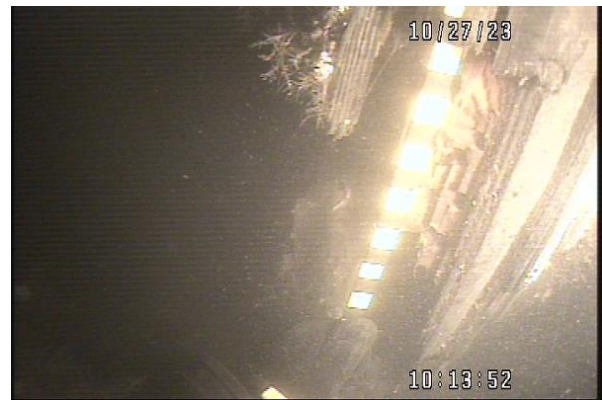
68. No. 2 pile cluster – NW pile – severed and with heavy worm tracks
