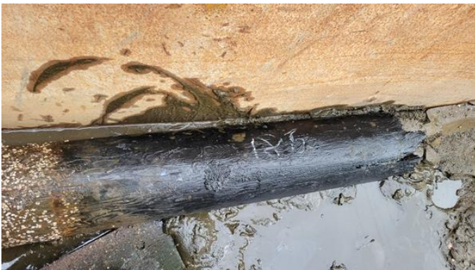
138. Pile 18 batter pile – broken off below mudline
