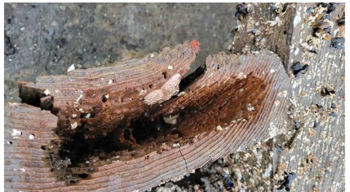
147. Pile No 20 horizontal support with core loss.
