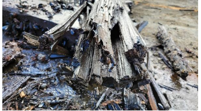
205. Pile cluster No 1 top – timber deteriorated
