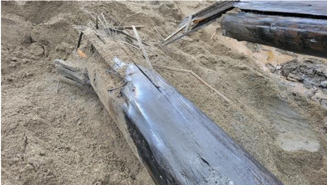
144. Pile No 20 – broken off below mudline
