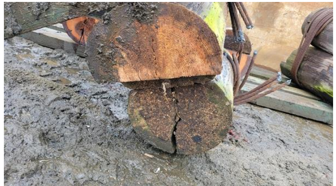
129. Top of Pile No. 26 – visually fair condition
