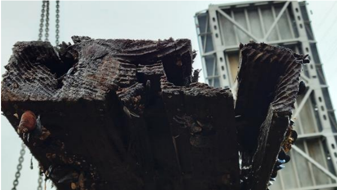
192. No 2 pile cluster – fender board with internal core degradation
