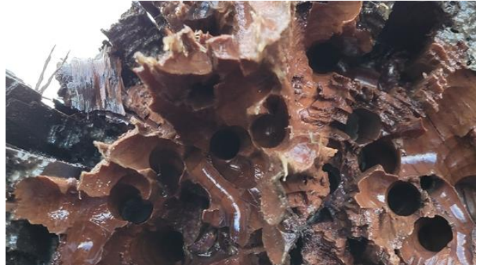
177. No 15 fender pile – broken with heavy core loss and worm tracks
