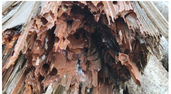
195. No 2 pile cluster – core degradation and worm tracks
