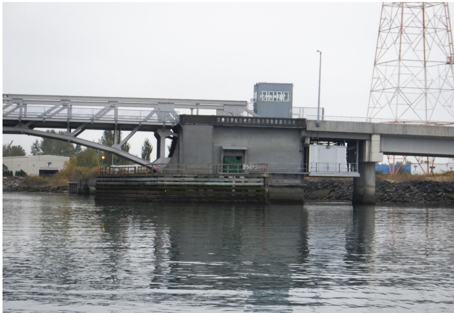
PHOTO No. 4 : Pier 3 and Pier 4, Looking Southeast - Note Pier 3 supported by two concrete columns and Pier 4, the Bascule pier, both located on the west side of the channel. Also note the protective timber fender system along the channel side of Pier 4.
