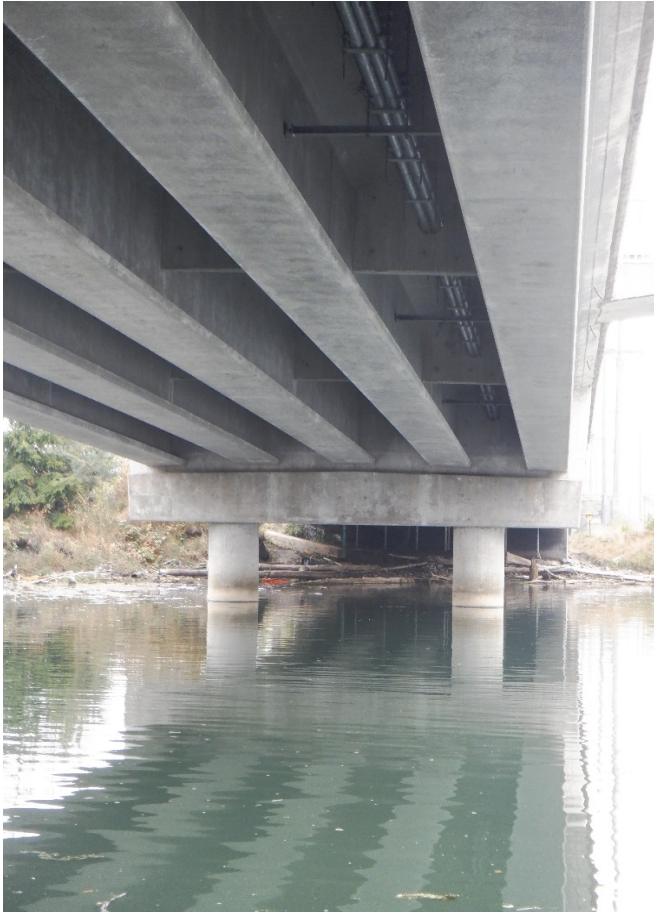
PHOTO No. 3 : Pier 2, Looking Southwest - Note the overall good condition of the concrete columns, beam and prestressed girders. Inspection of the columns found them to also be in overall good condition below water.
