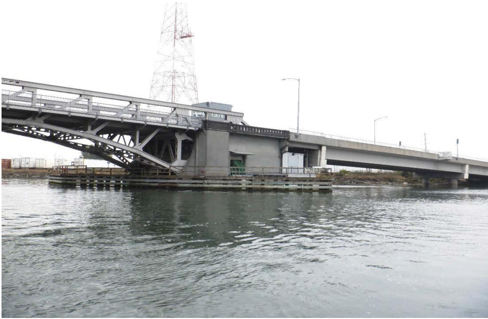
PHOTO No. 11 : Pier 4, Looking South - Note the protective timber fender system located along the channel side of the bascule pier. Although areas of fungal decay and marine borer damage were found, the overall condition of the system was found to be fair to good.
