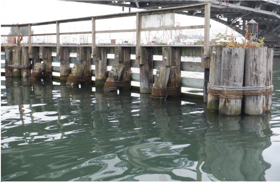
PHOTO No. 13 : Pier 5 Fender System, North End - Note the vegetation located in the tops of the dolphin piles. Also note the fair condition of the wire rope cable connections and the newer Chemonite Treated horizontal lagging.
