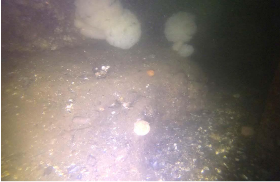
PHOTO No. 9 : Pier 4, Channel Side - Inspection found the top of the seal pour to be exposed along the channel side of the pier. Note the generally good condition of the seal and the silty-sand and shell which comprises the mudline at this location.
