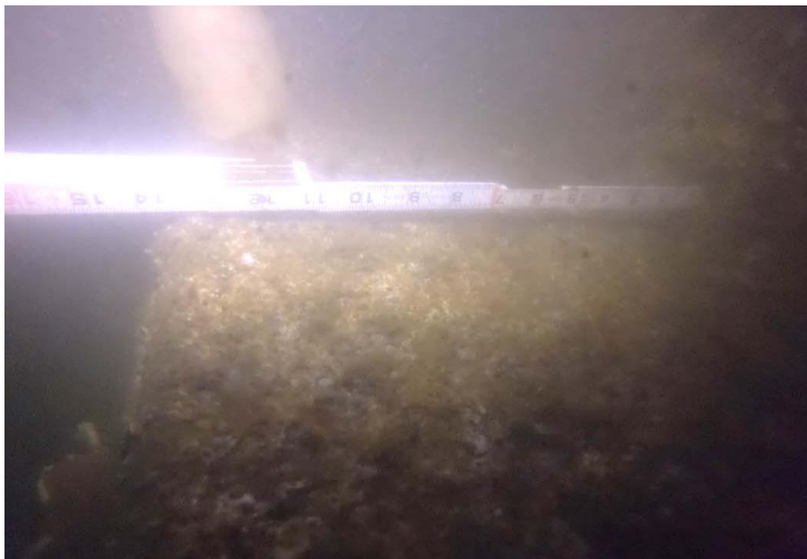
PHOTO No. 8 : Pier 4, Channel Side - Inspection of the bascule along the channel side found exposure of the footing and a portion of the seal pour. Note the overall fair condition of the top of the exposed concrete footing.
