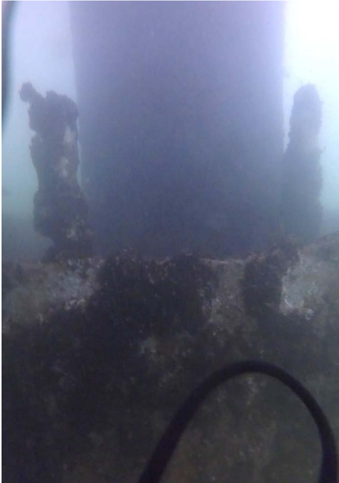
PHOTO No. 7 : Pier 3, North Column - Note the transition between the lower steel shaft and the upper concrete column. Inspection found the column to be in good condition with no significant damage noted to the concrete and minor surface corrosion of the lower steel shaft.
