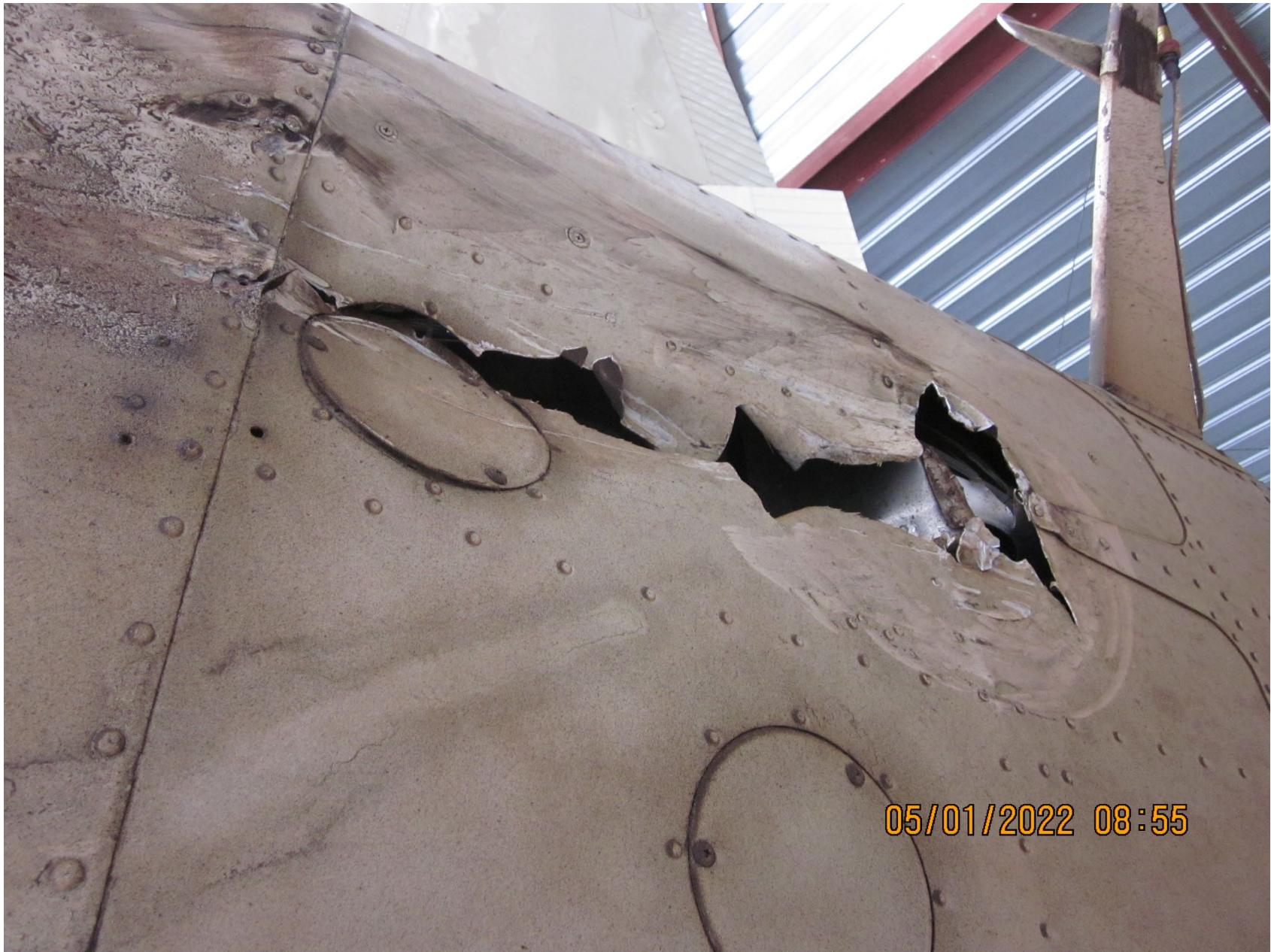
Photo 4 – Lower Fuselage (FAA Photo)
