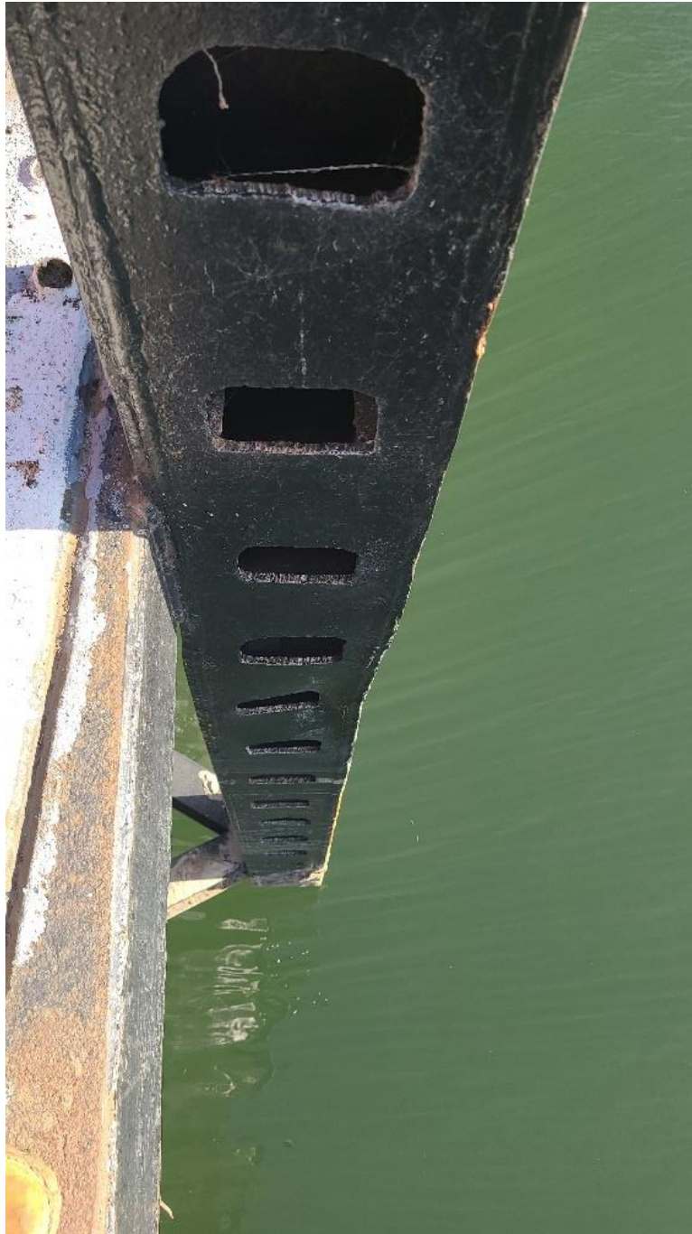
Starboard pushknee damage, looking down from above
