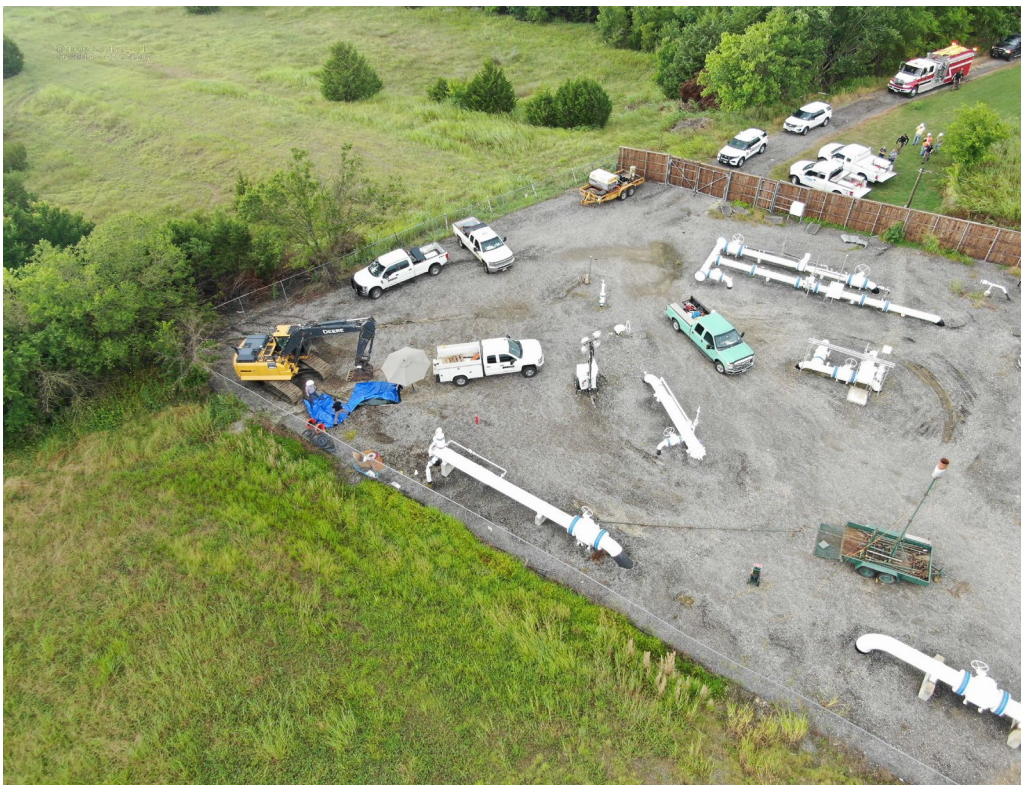
Figure 1: Accident Scene Photograph on June 28, 2021 (Courtesy of Wylie Fire Department)
