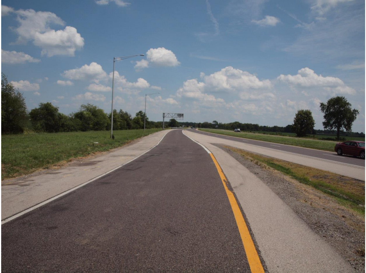
Highway Factors Photo 6 – View of the exit ramp to the westbound Silver Lake rest stop immediately west of the crash location standing on the exit ramp looking to the east
