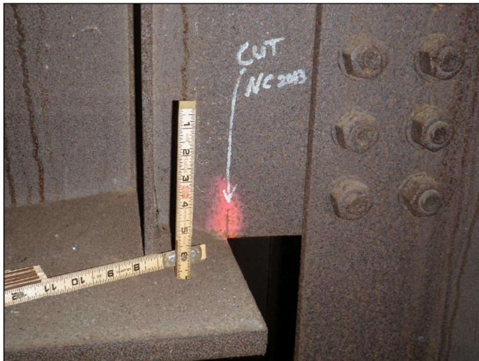
Photo 5 – Location of Fracture-Critical Members. Cut-short floorbeam flange at girder connection (AASHTO Fatigue Category E (Equivalent)). Floorbeam was over-cut when fabricated).
