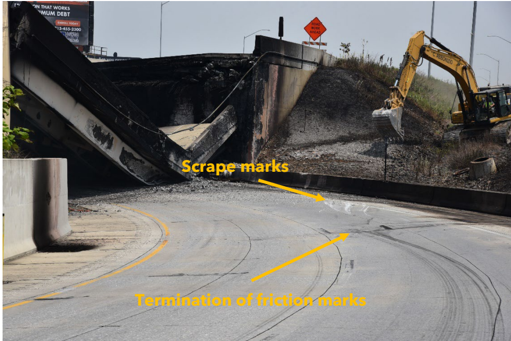
Figure 9. Photograph looking north along the Cottman Ave. off-ramp. The image shows the termination of the curvilinear friction marks. (Photo courtesy of PSP)
