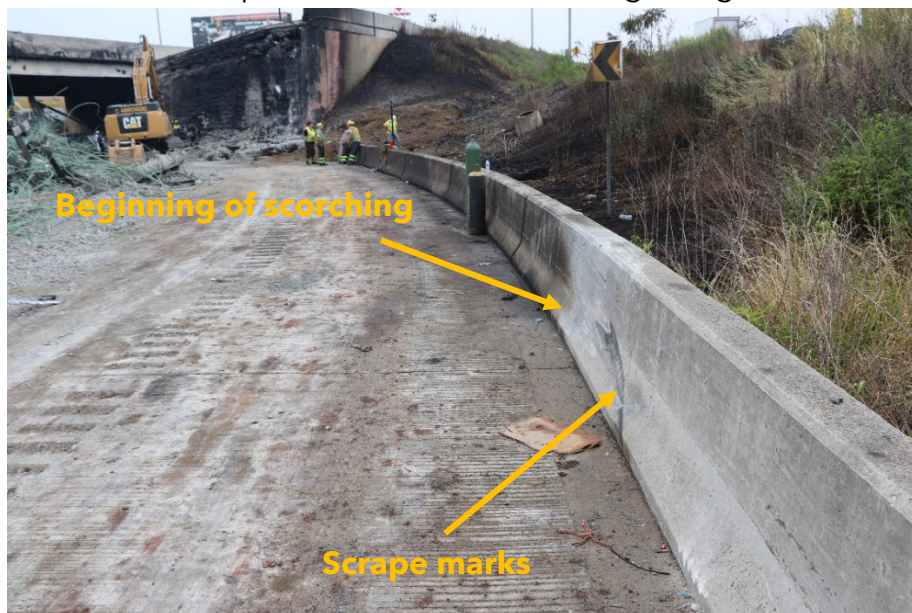
Figure 7. Photograph depicting the impact marks and scorching on the concrete barrier.
