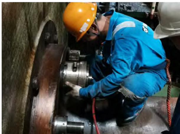
Removed FWD coupling bolts
