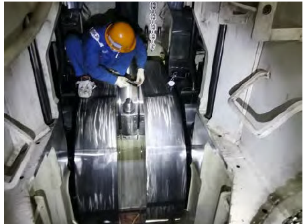
No.7unit FWD & AFT main bearing
