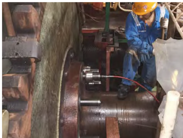
Removed FWD coupling bolts
