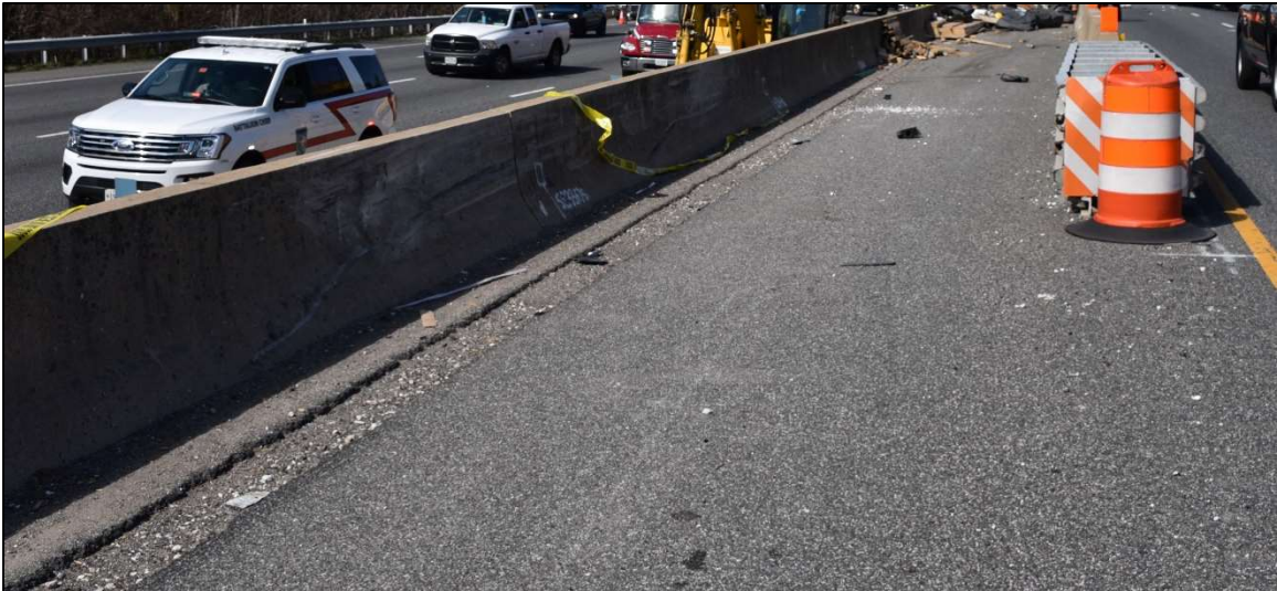
Figure 5: Impact damage to median barrier following Acura contact. (Maryland State Police (cropped))
