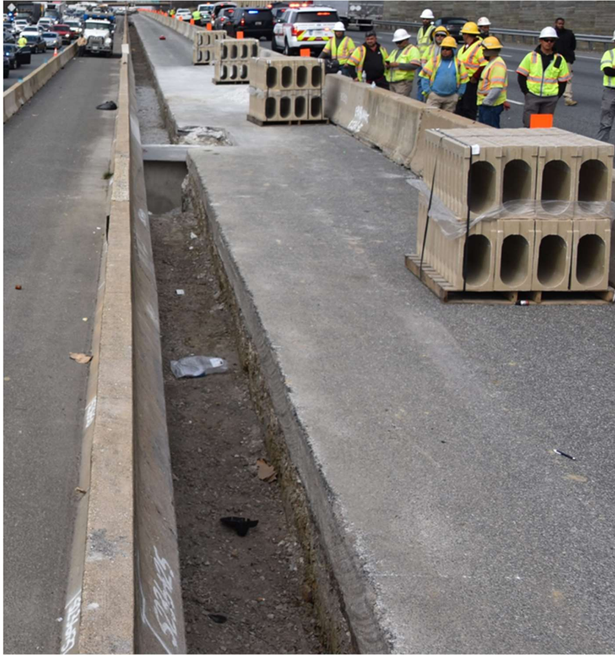
Figure 8: Photograph depicting exemplar storage of drain pallets within the work zone. (Maryland State Police - cropped)
