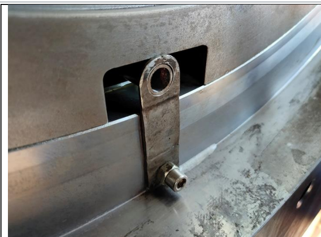
Fixed sampling pipe after side.
