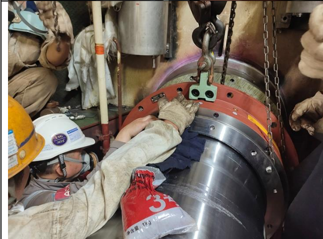
Mounted stern tub forward seal onto propeller shaft supervised by SKF's engineer.
