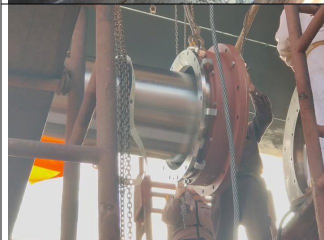
Mounted after stern tub seal onto propeller shaft supervised by SKF's engineer.
