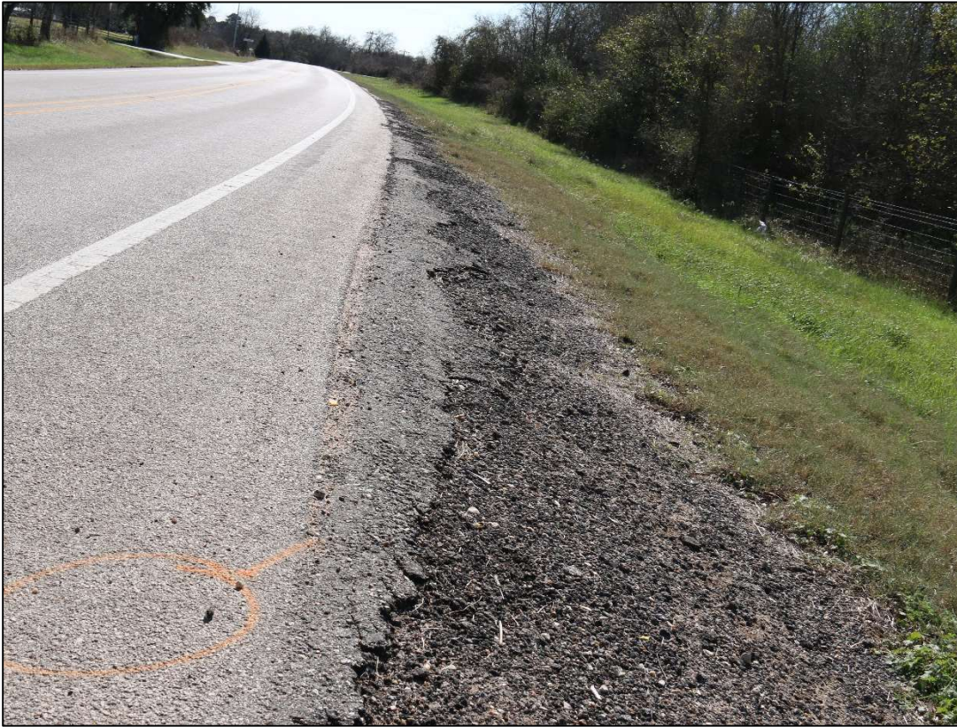
Figure 3: Photograph depicting southbound right roadway edge near area of bus roadway departure.
