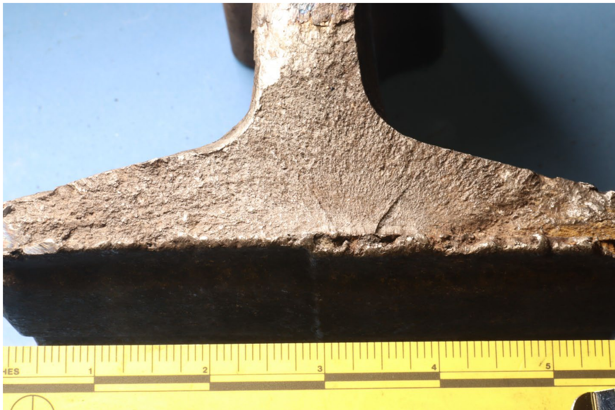
Figure 12. Angled view of the fracture initiation area of the downstream rail fracture 'A'.
