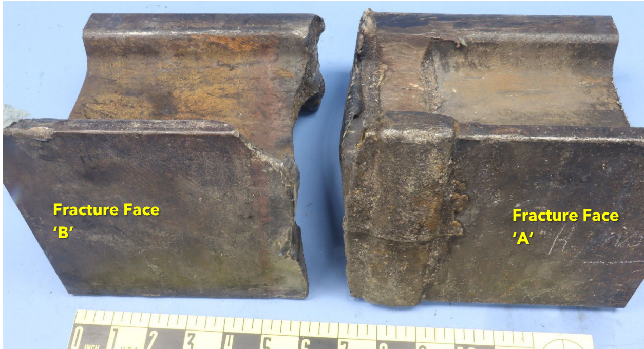
Figure 11. Angled view of the base underside from the field side of the fractured rail.
