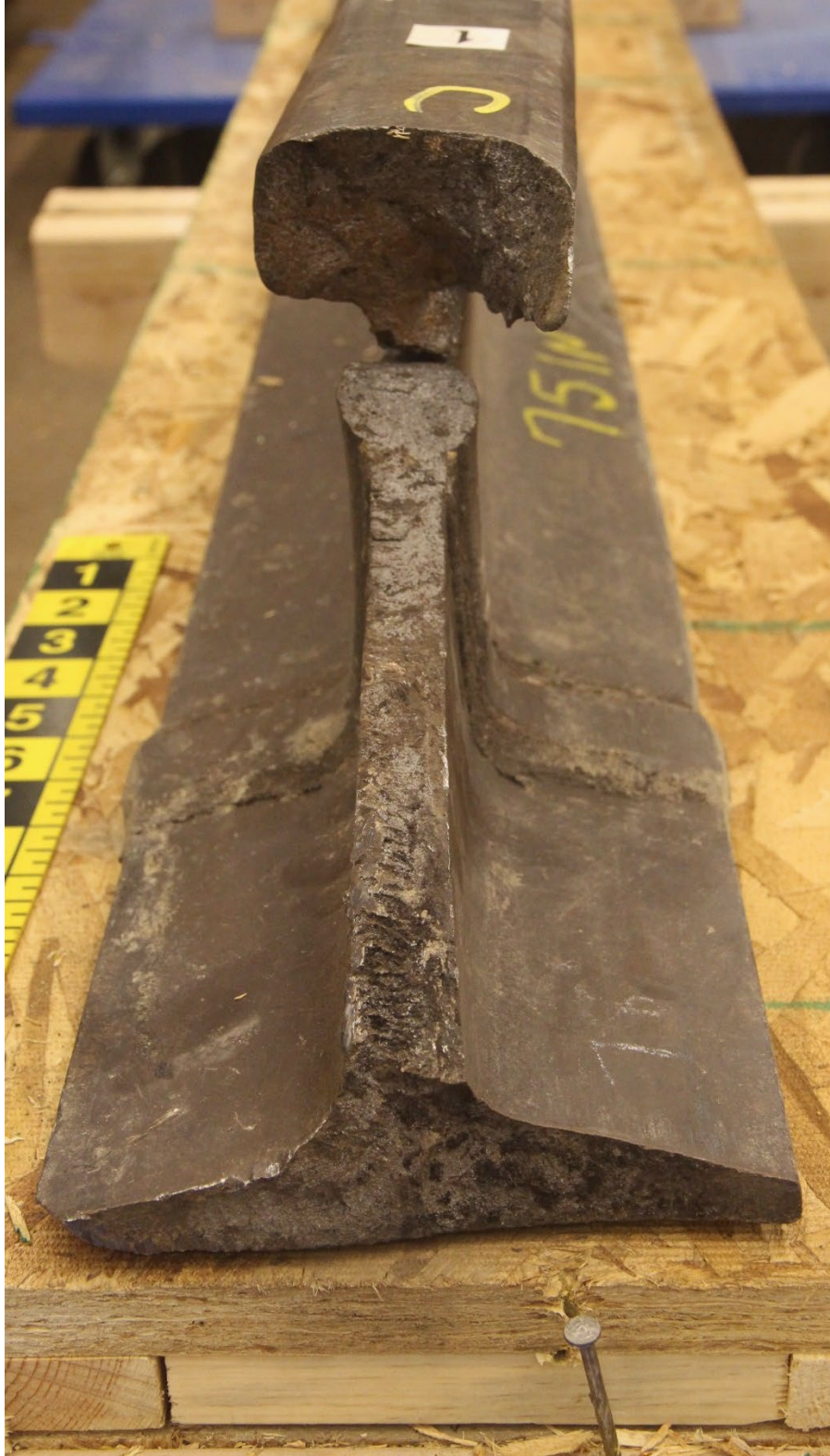
Figure 24. View of the second fracture surface through rail 3, showing from fracture surface 'C'.
