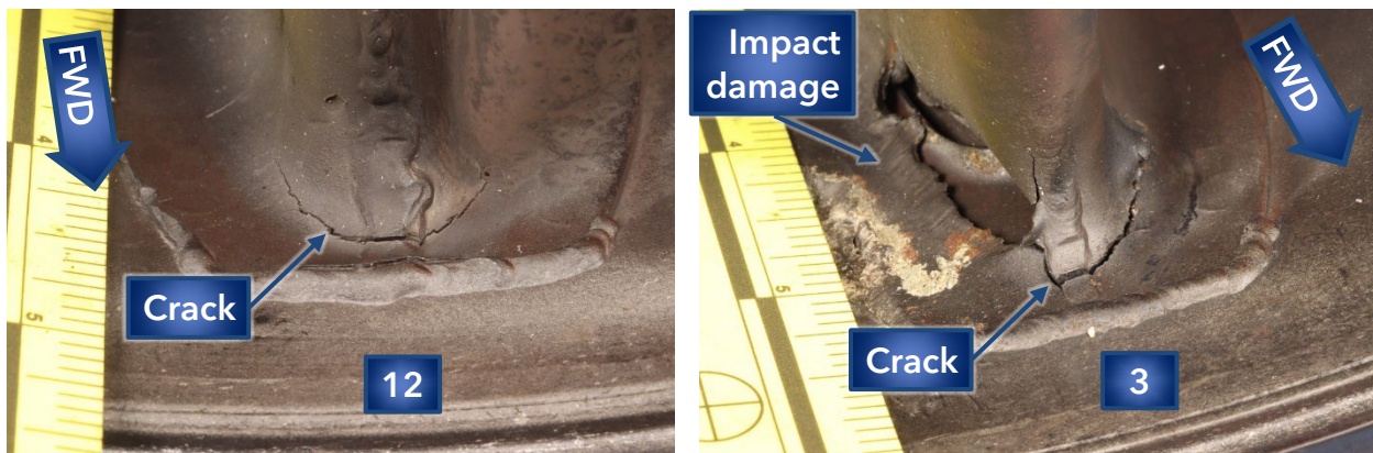
Figure 21. Cracks at the leading edges of two outer struts where they attached to the mid cone at the 12 o'clock and 3 o'clock positions.
