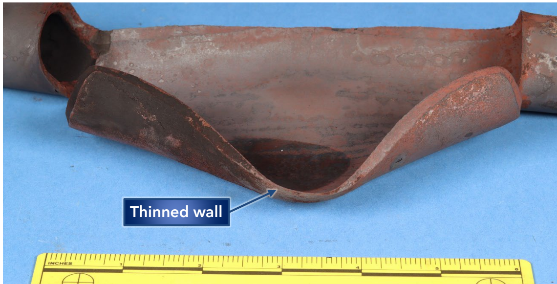
Figure 4. View from the lower side of pipe A showing wall thinning at the center of the bulge in the fracture location.
