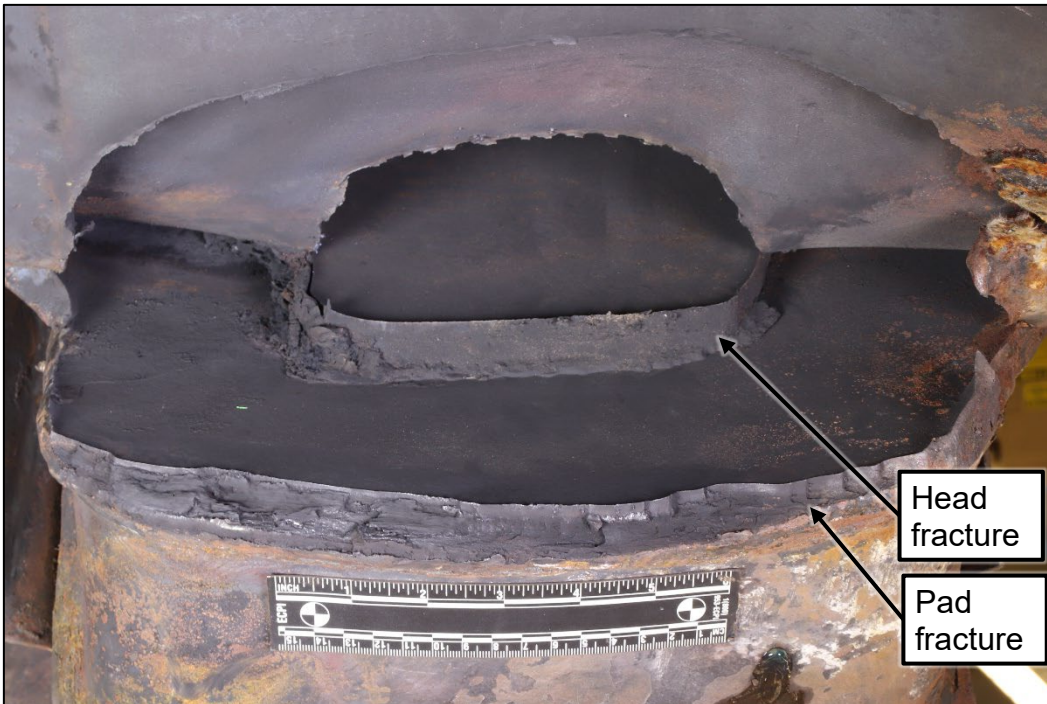
Figure 5. Closer view of fractures through the front sill pad and the head.
