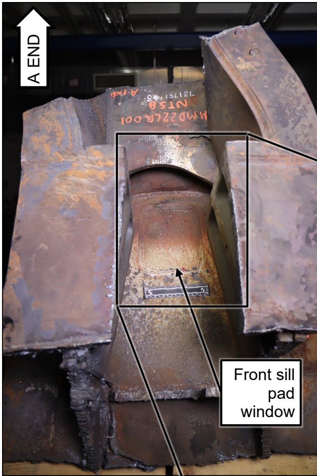
Figure 2. Lower side of the submitted tank car piece including a closer view of head brace-to-pad welds and pad-to-head welds at the front sill pad window (area where head is visible).
