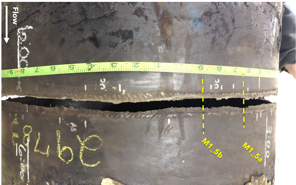
Figure 4. View of the mating fractured of Pipe 1 and 2 between the 6 and 3 o'clock positions, annotated to show metallographic mount locations and girth weld flaws: arc strike (AS) and undercut (UC).
