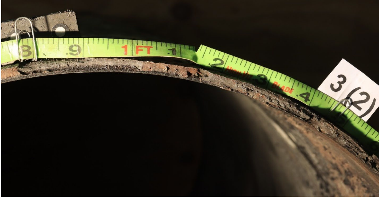
Figure 27. View of the Pipe 2 fracture surface counterclockwise of the 3 o'clock position.
