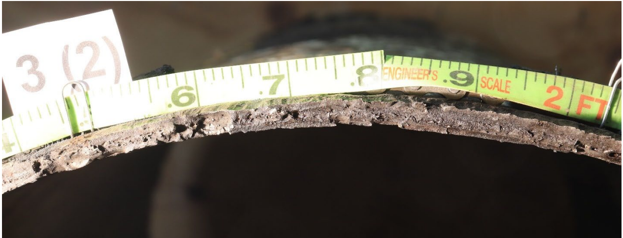
Figure 28. View of the Pipe 2 fracture surface clockwise of the 3 o'clock position.
