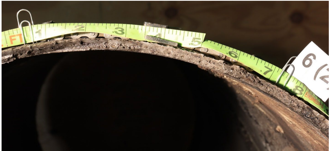
Figure 30. View of the Pipe 2 fracture surface counterclockwise of the 6 o'clock position.
