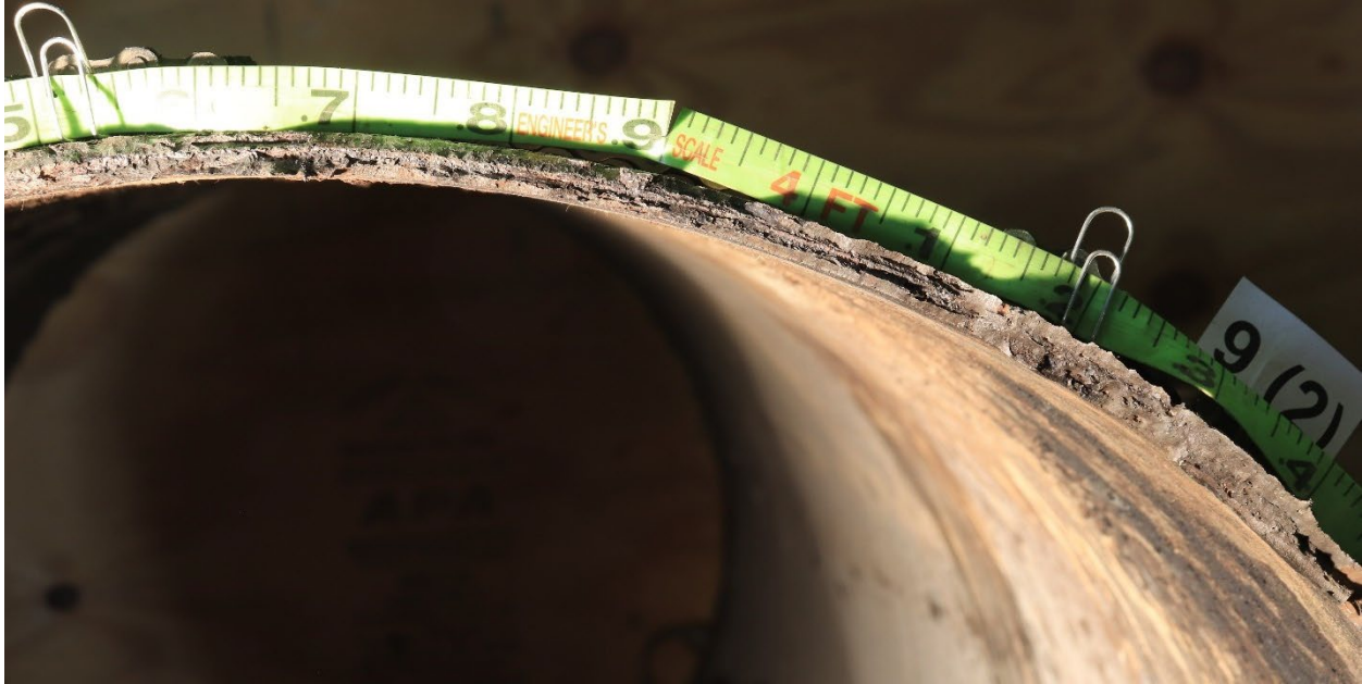
Figure 31. View of the Pipe 2 fracture surface counterclockwise of the 9 o'clock position.
