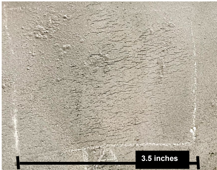
Appendix 2D. Outer surface of region 1A when viewed with incandescent light showing surface breaking cracks that coincided with colonies of longitudinal crack indications. Photograph taken after grit blast cleaning and MPI. Pitting corrosion is present in the general area.
