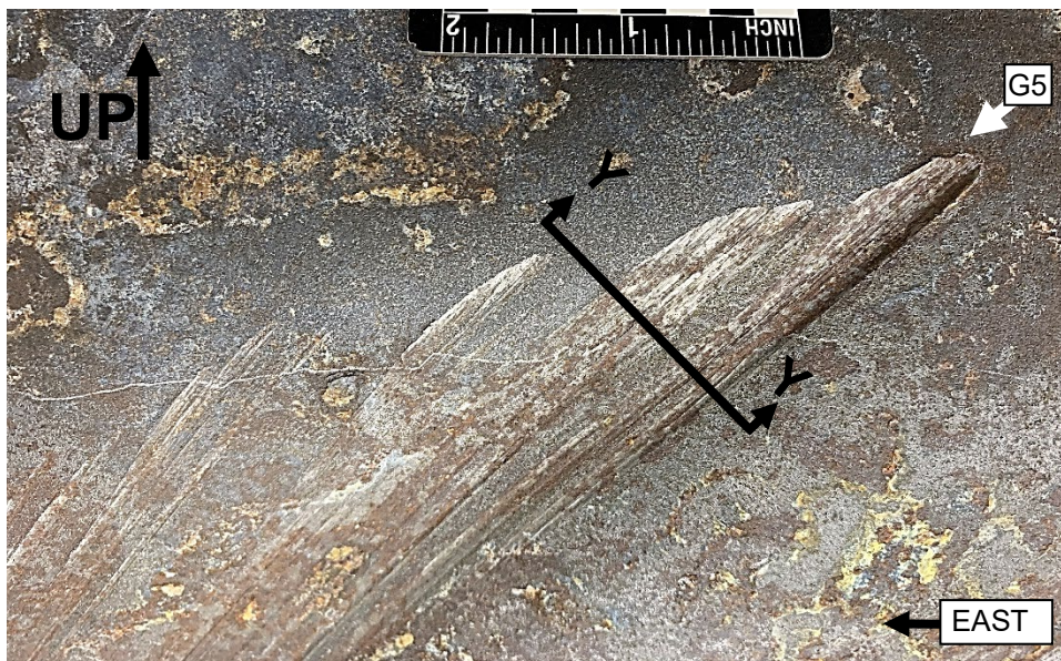
Figure 15. Close-up photograph of the outer surface of the pipe in the area of elongated dent “G5” showing several gouges at the upper end of the elongated dent, after cleaning.
