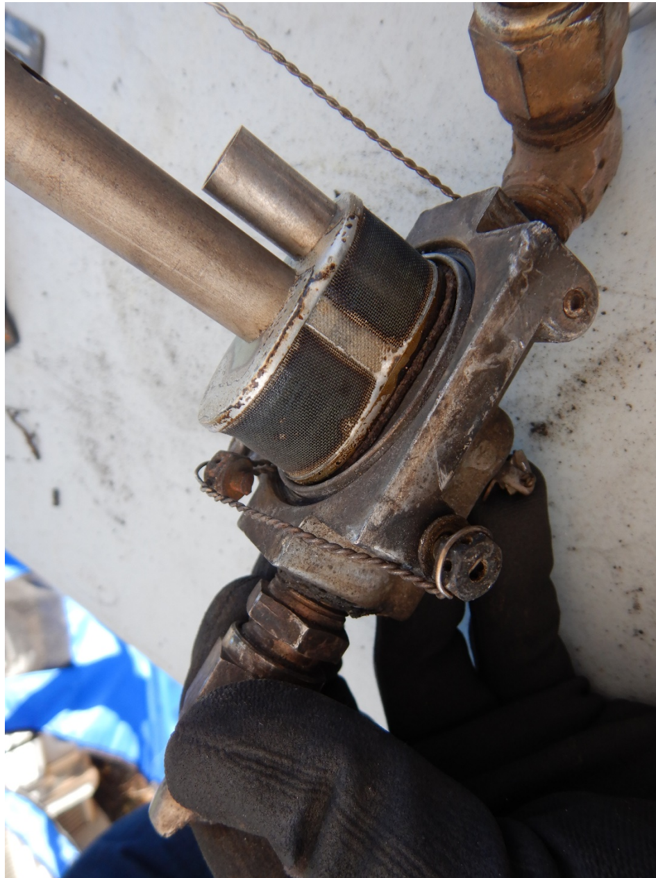
Photo 29 - Supplied close-up photo of gascolator fuel filter strainer screen.
