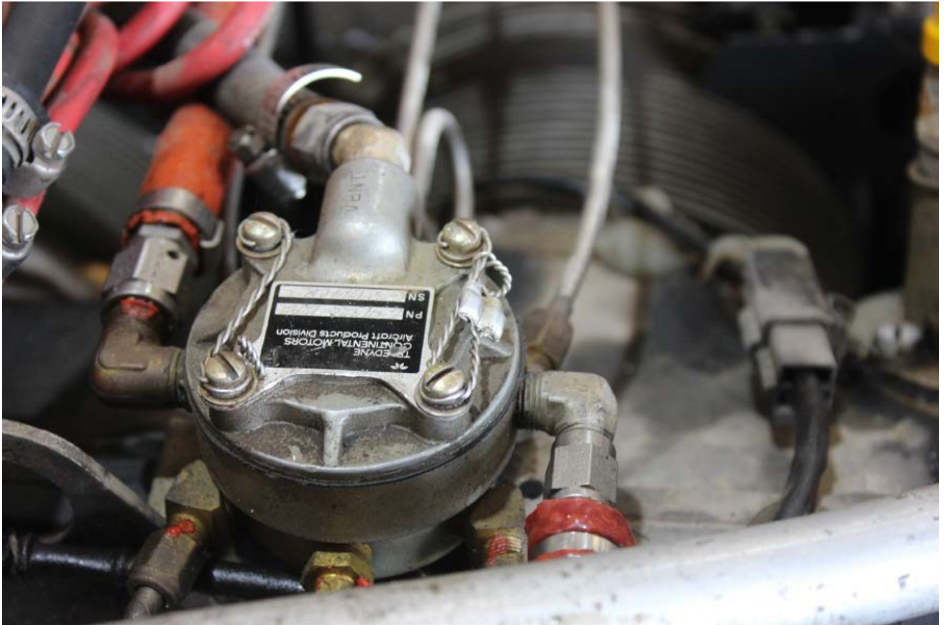
Photo 7 - Supplied close-up photo of the fuel manifold valve.
