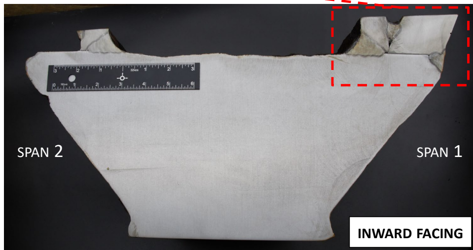
Figure 47. Cross-section through the span 1 side flange joint on the inward facing side. (Etchant: 5% nital) (Bottom two photos by FHWA)
