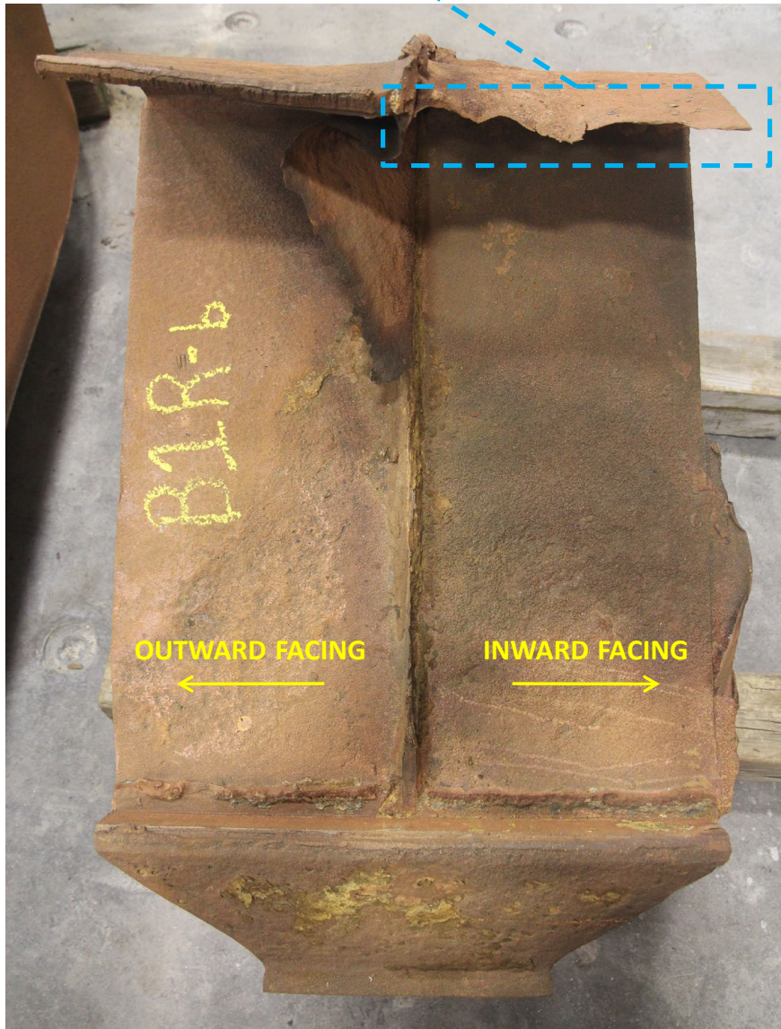
Figure 13. Photos of the end of the tie plate that separated from the span 2 side flange on the inward facing side of the leg.
