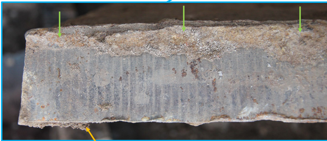
Figure 37. Close-up photos of the flange end on the bottom of the rolled span 2 side flange while it was still attached to the leg on-scene. The orange arrows point to remnants of the inner weld where the toe, flange end, and bearing stiffener mated and the green arrows point to remnants of the outer weld where the toe and flange end mated.
