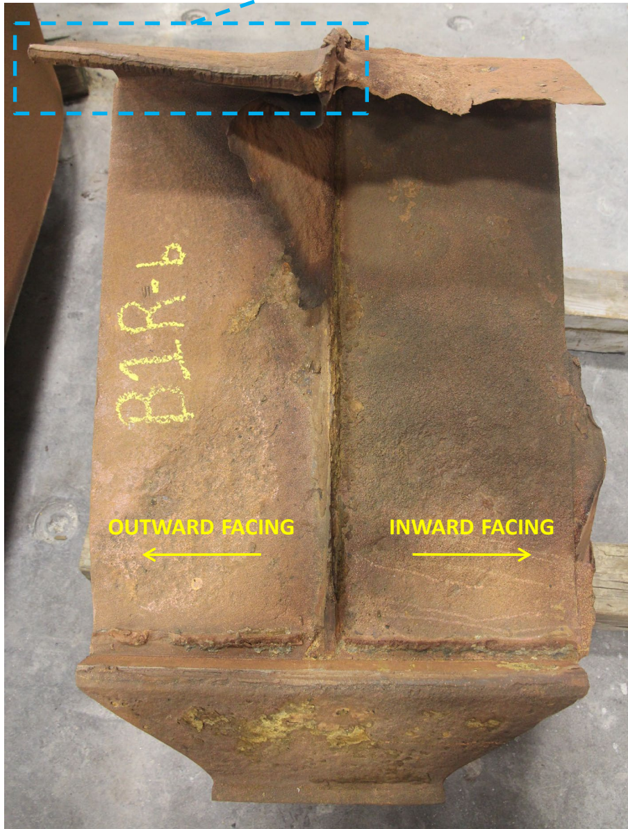
Figure 14. Photos of the end of the tie plate that separated from the span 2 side flange on the outward facing side of the leg. The white arrows point to weld material still joined to the plate faces.
