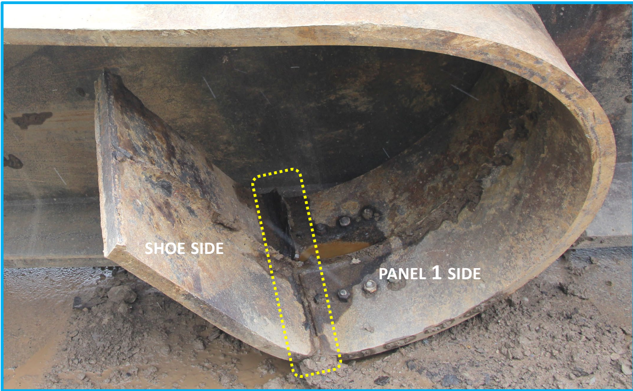
Figure 15. Photos showing the top half of leg B1R with the separated span 2 side flange rolled up on the outward facing side of the leg. The yellow dotted line encircles the location on the internal surface of the span 2 side flange that mated with the tie plates.
