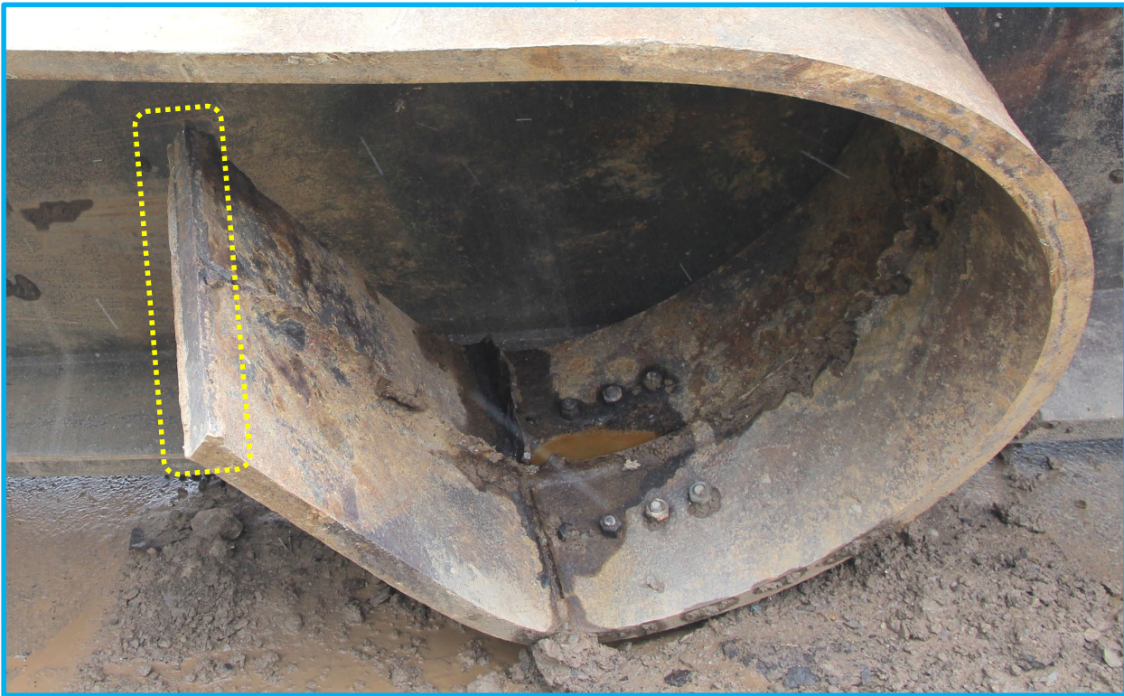
Figure 36. Photos of the bottom of the rolled span 2 side flange while it was still attached to the leg on-scene. The yellow dotted line encircles the flange end.
