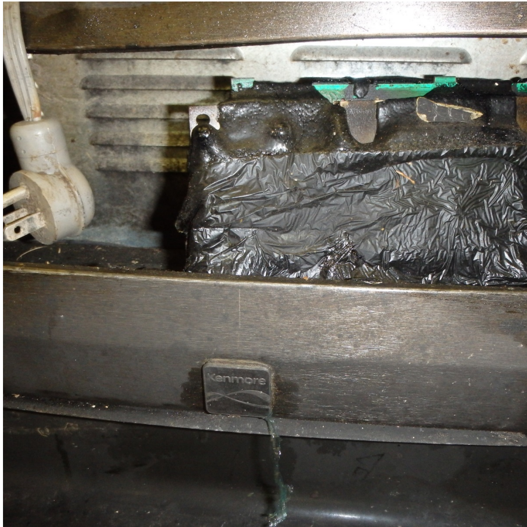
Figure 48. Control panel of 3515 Durango Drive gas range. Photograph by DFR, June 2020.
