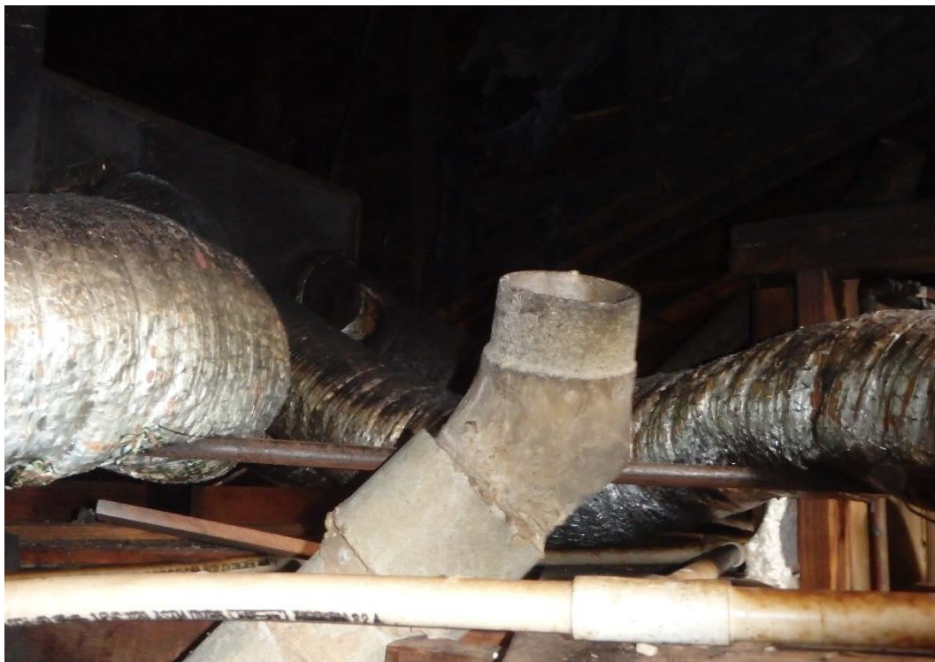
Figure 18. Damage to ducting in attic of 3527 Durango Drive. Photograph by DFR, February 2018.
