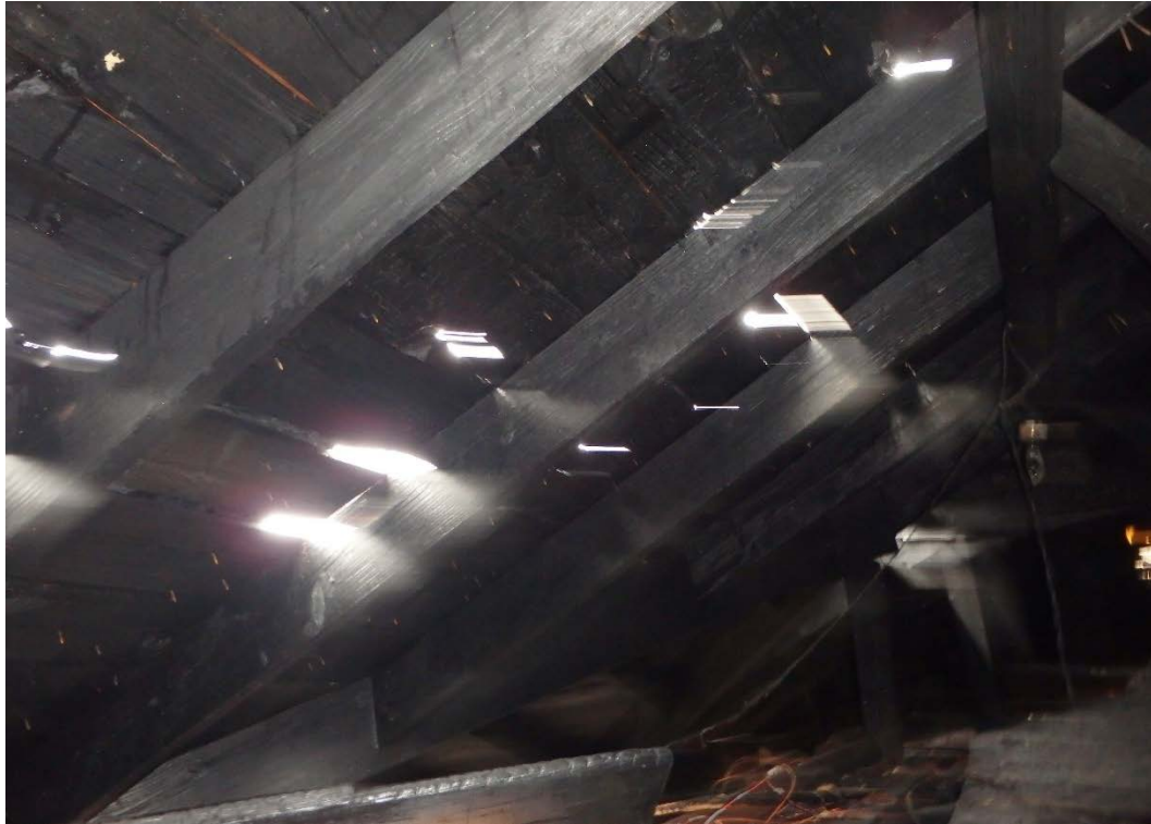
Figure 17. Damage to attic and roof structure in 3527 Durango Drive. Photograph by DFR, February 2018.
