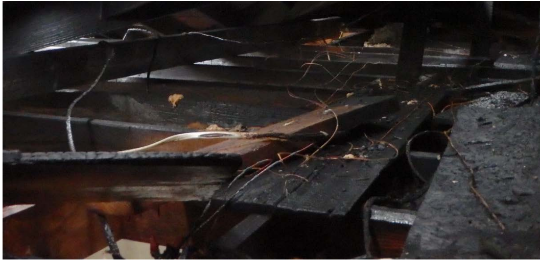
Figure 19. Damaged wiring and attic structure in 3527 Durango Drive. Photograph by DFR, February 2018.
