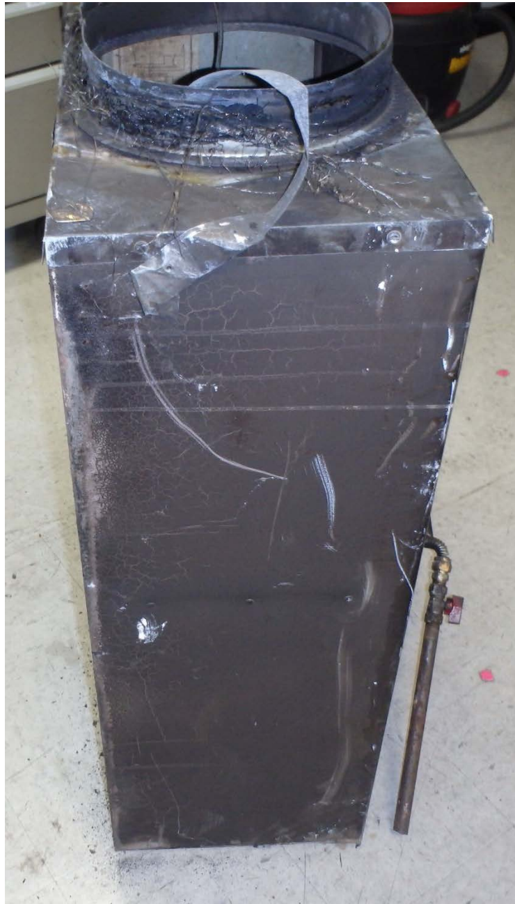
Figure 30. Furnace unit from 3527 Durango Drive (Side B). Photograph by DFR, June 2020.
