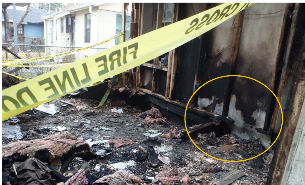
Figure 21. Closeup of calcination (highlighted with yellow circle) on wall in addition bedroom for 3527 Durango Drive. Photograph by DFR, February 2018.
