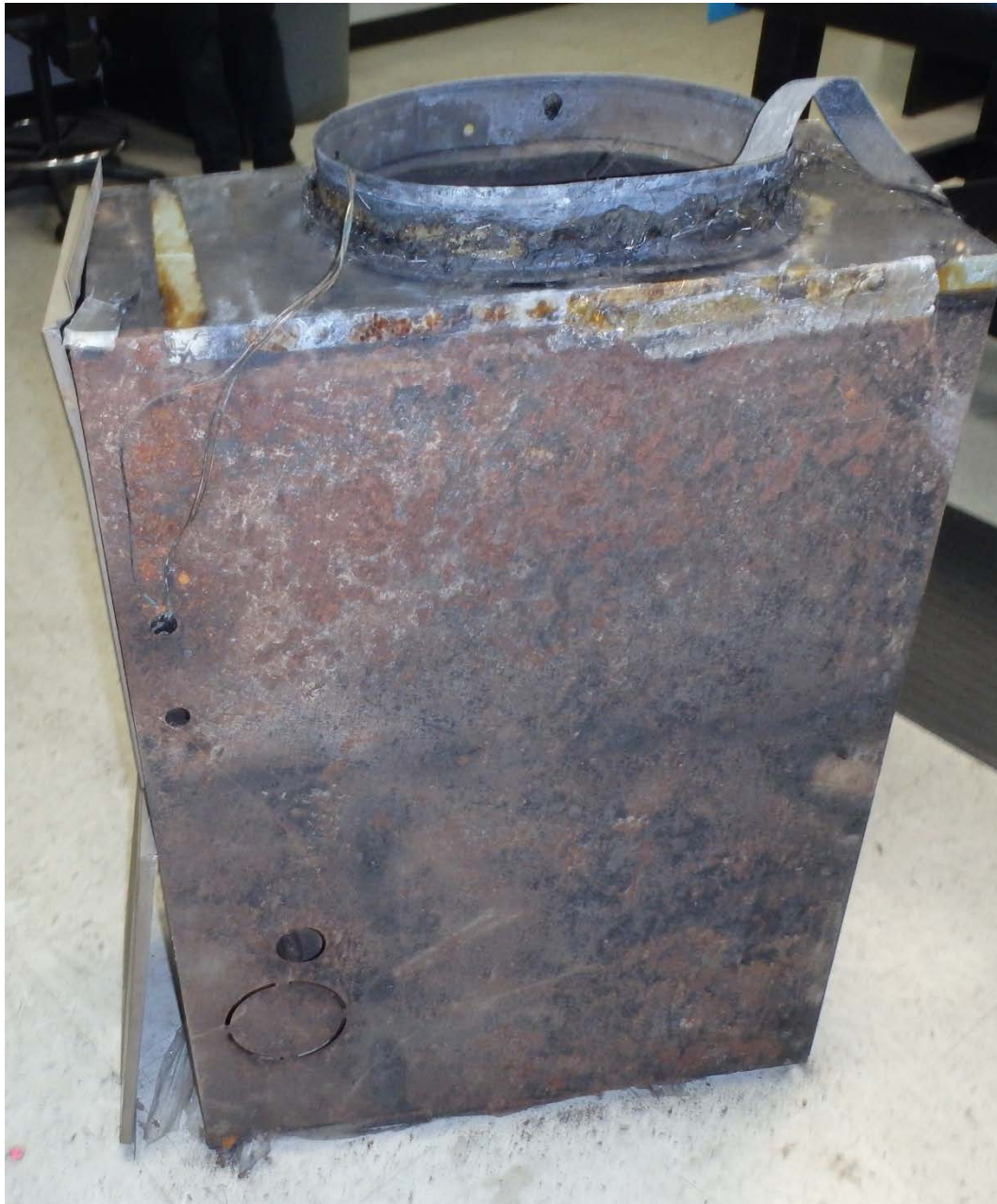
Figure 29. Furnace unit from 3527 Durango Drive (Side A). Photograph by DFR, June 2020.
