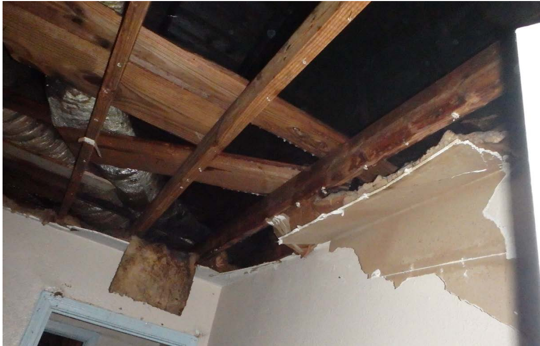
Figure 14. Closeup of ceiling rafters in living room of 3527 Durango Drive. Photograph by DFR, February 2018.
