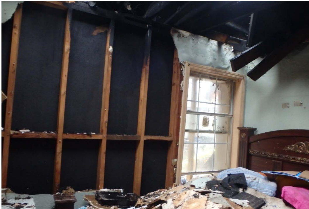
Figure 15. Bedroom wall between original structure and addition in 3527 Durango Drive. Photograph by DFR, February 2018.
