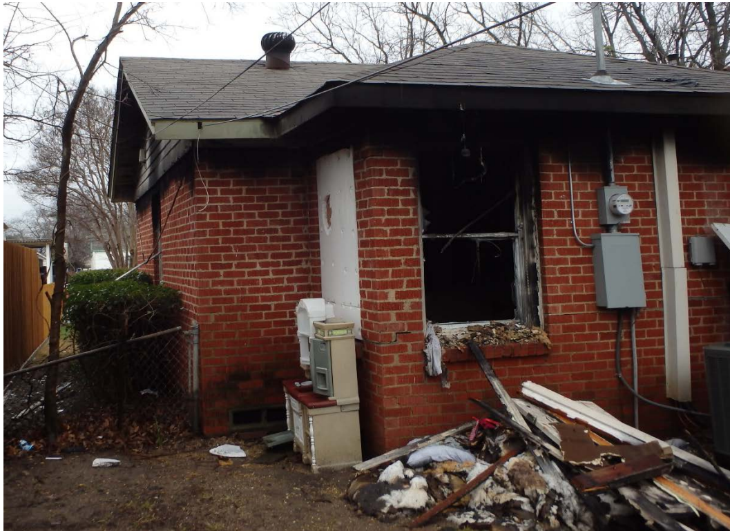
Figure 40. Corner of Side C and Side D of 3515 Durango Drive. Photograph by DFR, February 2018.
