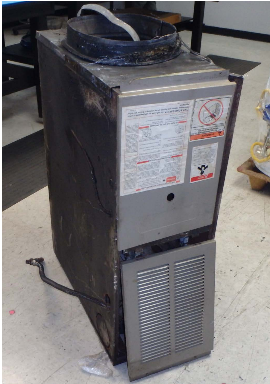
Figure 32. Furnace unit from 3527 Durango Drive (Side D). Photograph by DFR, June 2020.
