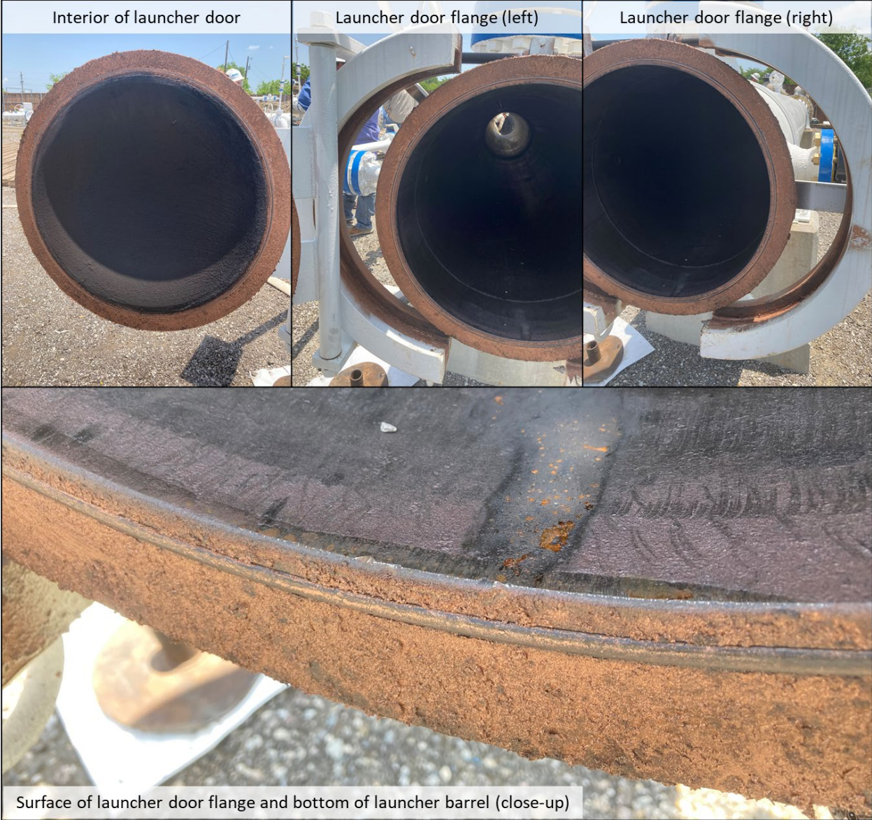
Figure 8. Corrosion on launcher door mating surfaces, July 13, 2021 (Courtesy of RRC)
