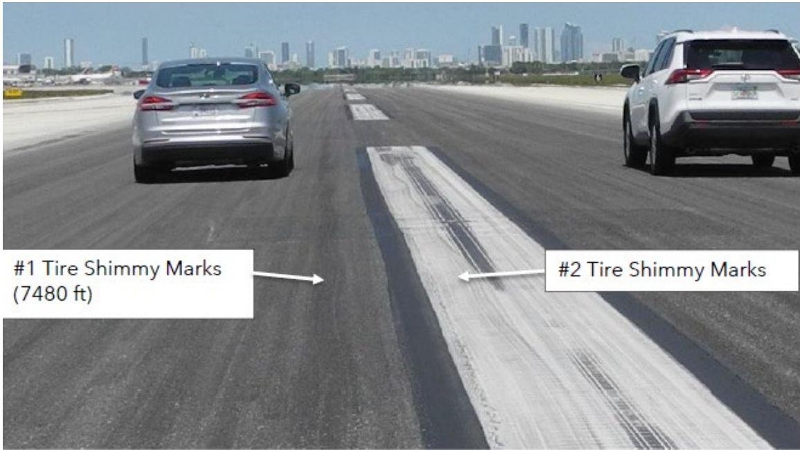
Figure 2 Start of left main gear shimmy marks
