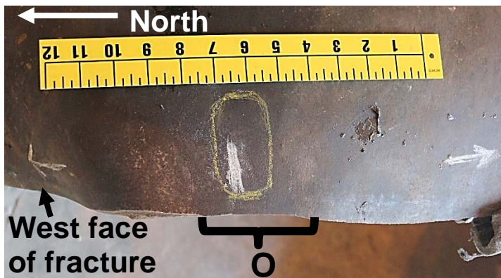
Figure 7. Photograph of the outer surface of the pipe at the west face of the fracture (fracture face is facing down) showing the fracture origin area, indicated by bracket "O". The outer surface adjacent to the fracture origin exhibited an isolated area that was flat when a straight edge was placed perpendicular to the length of the pipe for the area enclosed by the yellow line, but the outer surface on the same area exhibited evidence outward bending deformation when a straight edge was placed parallel to the length of the pipe. The area marked in yellow measured approximately 2 inches along the length of the pipe and approximately 3 inches along the circumference.
