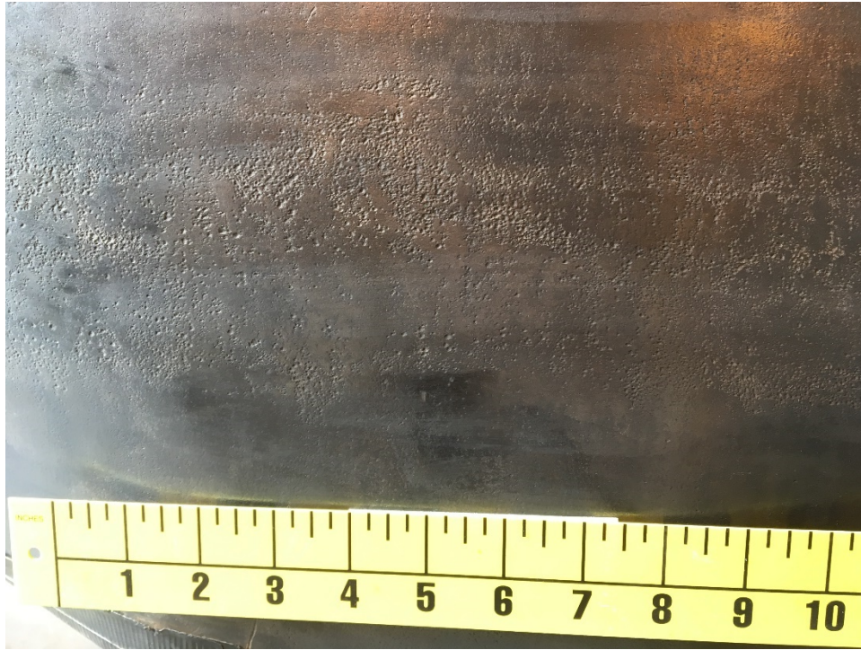
Figure 3: Zoomed View of Surface corrosion Pitting within East Inspection Area. Photo by NTSB
