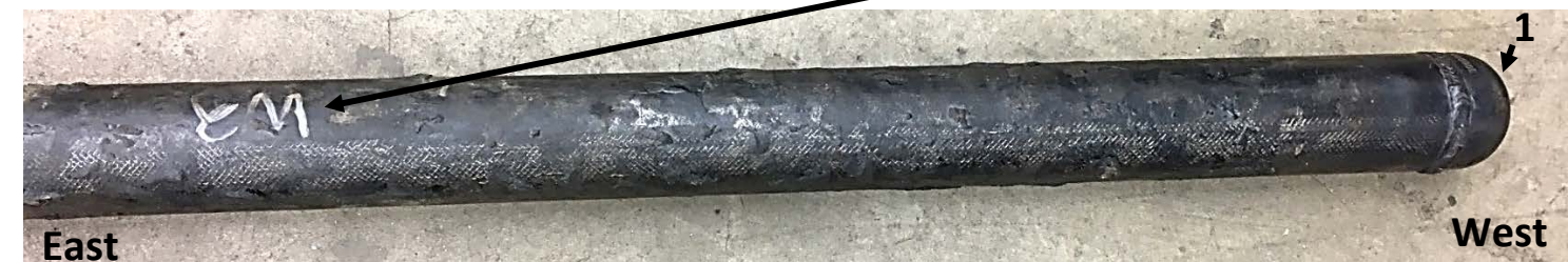
Appendix 4. Photographs of the 10-foot main segment of the main that was located behind dwelling 3539 Durango Drive showing exposed areas with damaged coating indicated by brackets "A", "B", "C", and "D". Saw cuts made by NTSB lab are identified by arrows "2" through "5". Field cut is identified by arrow "6". Weld cap end made on-site is indicated by arrow "1". Ring sections cut by NTSB lab and portions tested by Lehigh and Westmoreland laboratories are indicated on the top photograph. Area "B" contains the dent and crack. Dashed circle indicates location where a longitudinal saw cut was made by NTSB lab through the main causing the top half of the main to separate from the bottom half and exposing the crack that intersected dent "B". Refer to NTSB Materials Laboratory Factual Report No. 18-067 for photographs of the as-received main segment.
