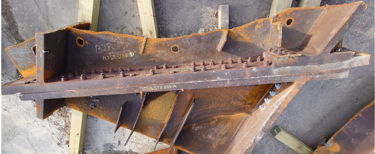
Figure A.26. B2R – NTSB-STR-028A (Taken at TFHRC).
