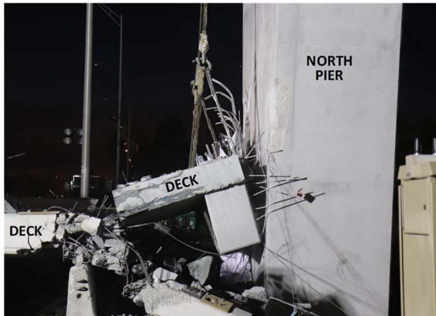
Figure 6: Photos looking west showing jackhammering and removal via crane of the large deck piece.
