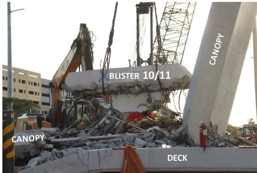
Figure 2: Photos looking west showing the removal via crane of Diagonal 11 (top) and Blister 10/11 (bottom).
