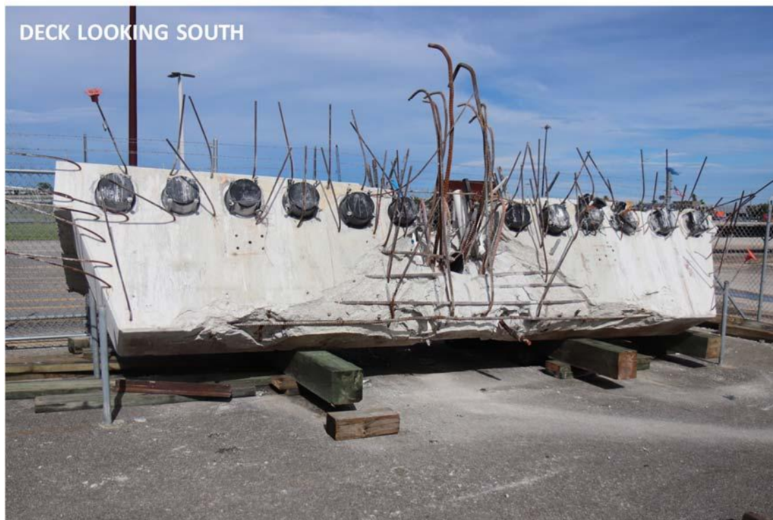
Figure 11: Photos showing the large deck piece after placement in the FDOT yard. Damage is visible on the north face of the deck. The locations of the large-diameter concrete cores that served as pick points for moving the piece are indicated.
