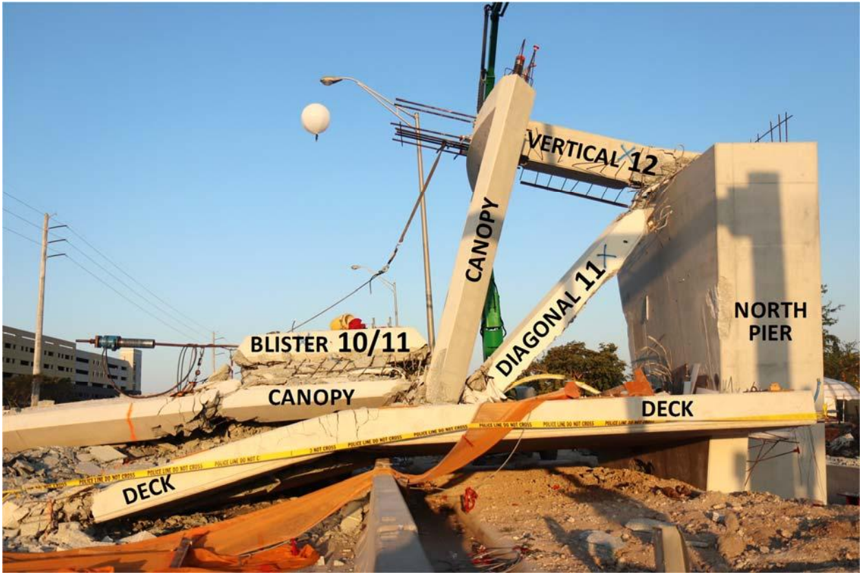
Figure 1: Photo looking west showing the north end of the bridge after collapse.
