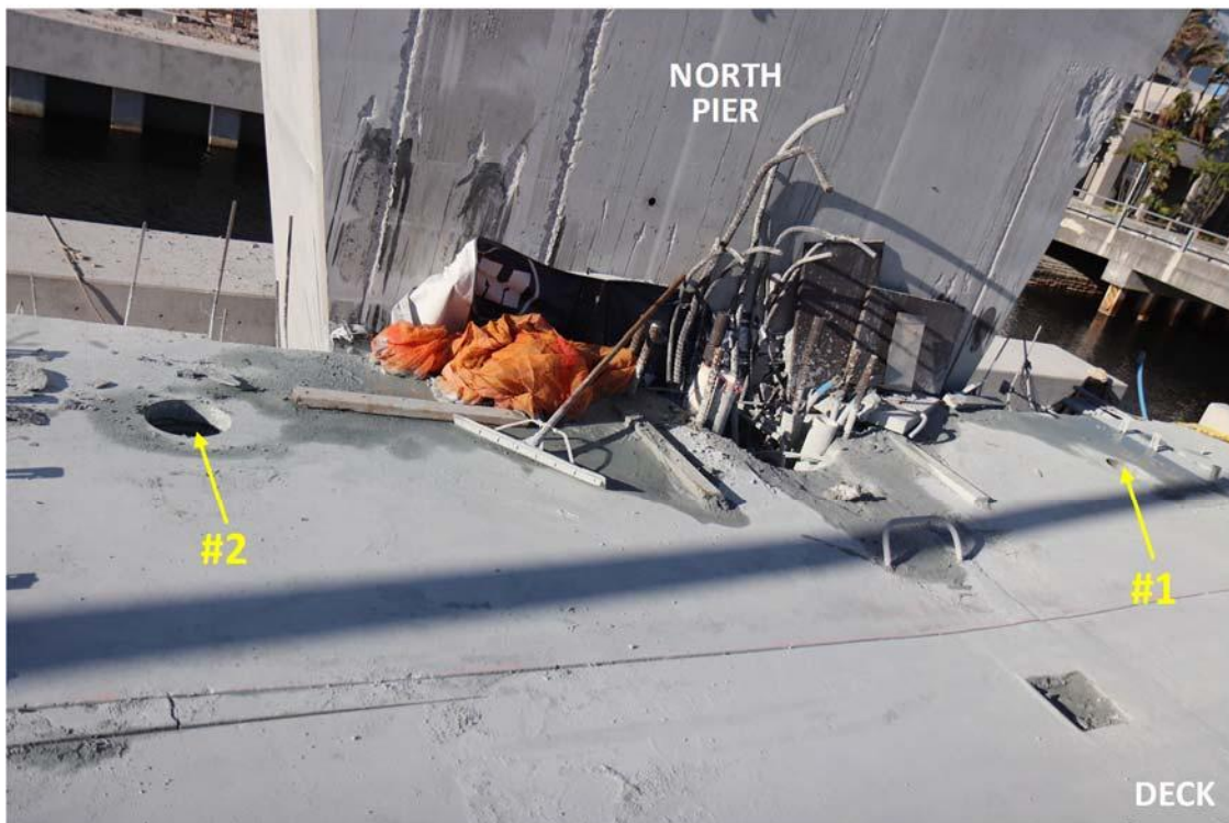
Figure 4: Photos showing the saw cut of the center two-thirds of the northmost portion of the deck. The two large-diameter cores taken to provide pick points for lifting the piece are indicated.
