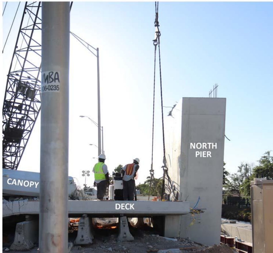
Figure 5: Photos looking west showing positioning of the crane for support and eventual removal of the large deck piece.
