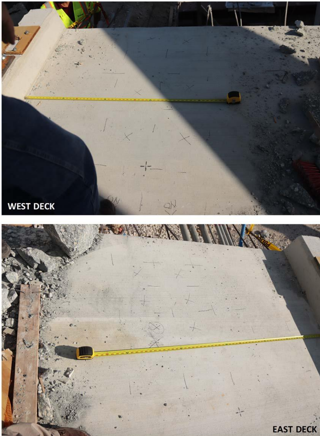
Figure 8: Photos showing the marked locations where concrete core samples for materials testing were taken from the east and west side of the deck. Per the design plans and ultrasonic inspection, the indicated areas were clear of underlying steel and plastic conduit internal to the deck.
