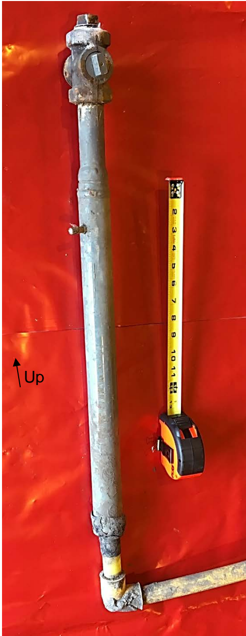
Figure 21. Close-up photograph of the as-received gas meter riser and portion of the service pipe.
