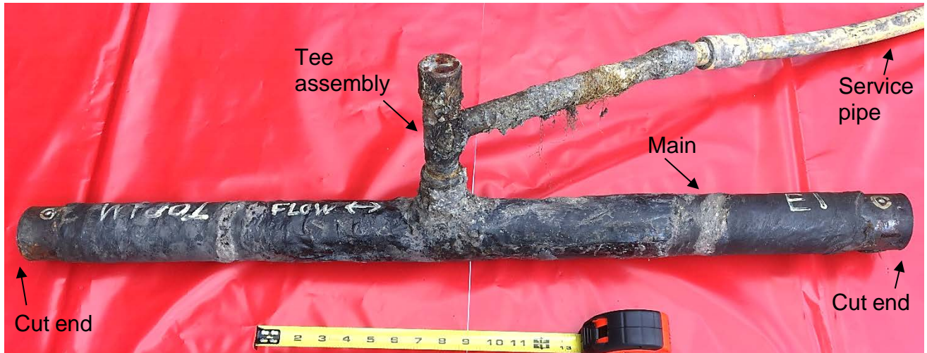
Figure 19. Close-up view of the Tee assembly and as-received portion of the main with the service pipe
