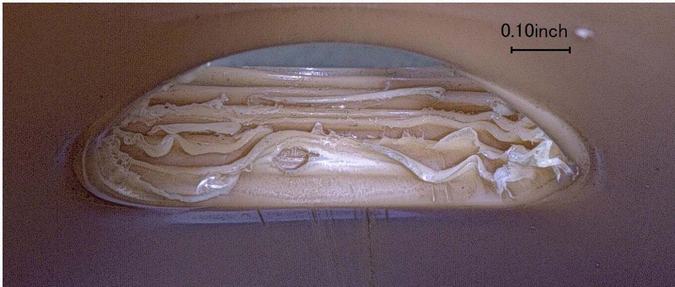
Figure 14. Photograph of the exposed inner surface of the main after the locking sleeve and tower of tee assembly "C" was forcefully pulled out of the main showing thread damage in the pierced hole.
