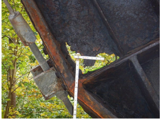
Figure A-2. Bent 1 right leg, inside face, far side, from the September 2021 report.
