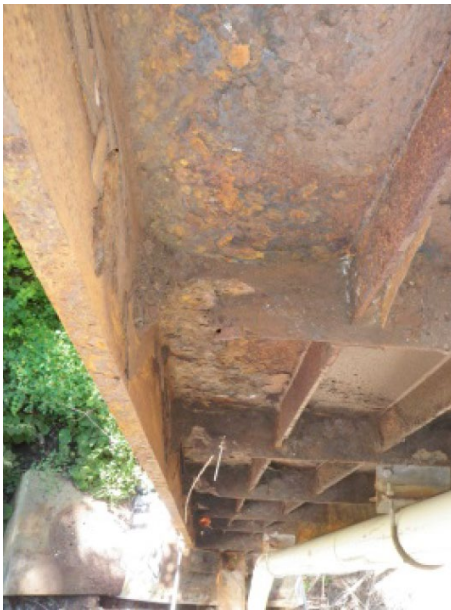
Figure A-3. Looking down Bent 1 right leg, inside face, from the September 2013 report.
