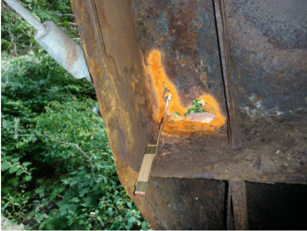
Figure A-1. Bent 1 right leg, inside face, far side, from the September 2013 inspection.
