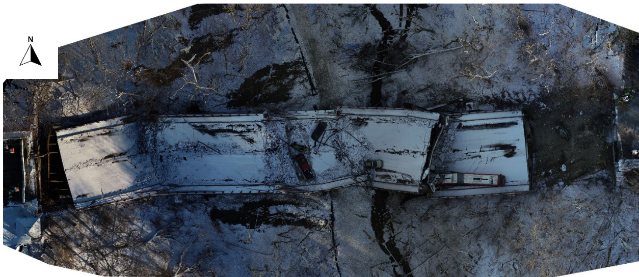
Figure 6. Drone image of collapse site.
