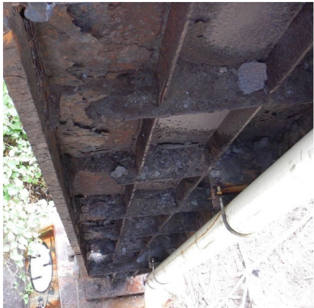
Figure A-4. Looking down Bent 1 right leg, inside face, from the September 2021 report.
