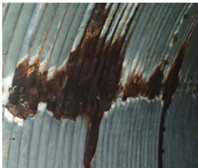
Figure IE 4.3.5.10-2 – Example of Corrosion and Section Loss Along Longitudinal Bolt Line
