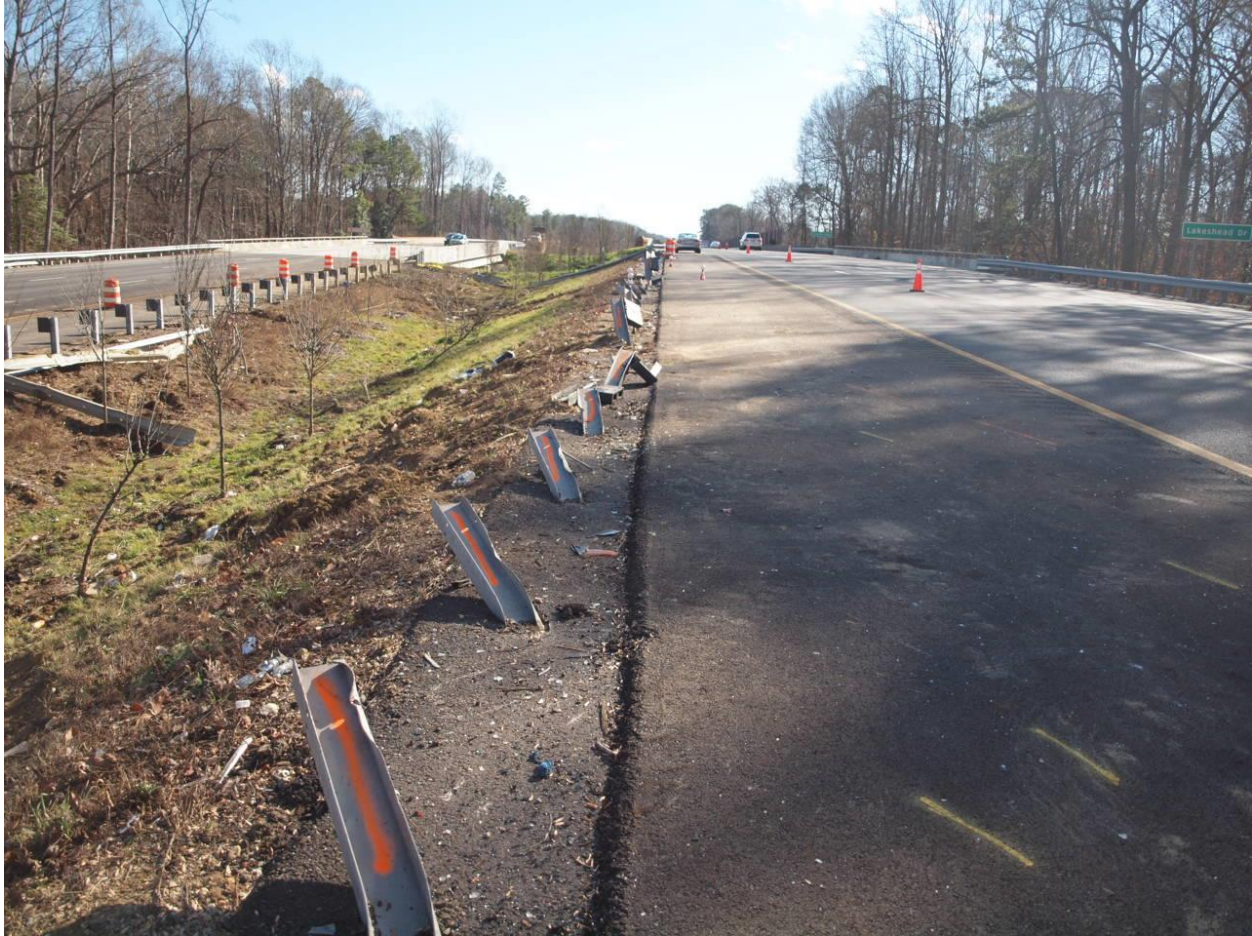
Highway Factors Photo 8 – View of deformed W 6 x 9 steel I-beam posts standing in the paved shoulder adjacent to the leftmost travel lane in the eastbound direction looking to the southeast
