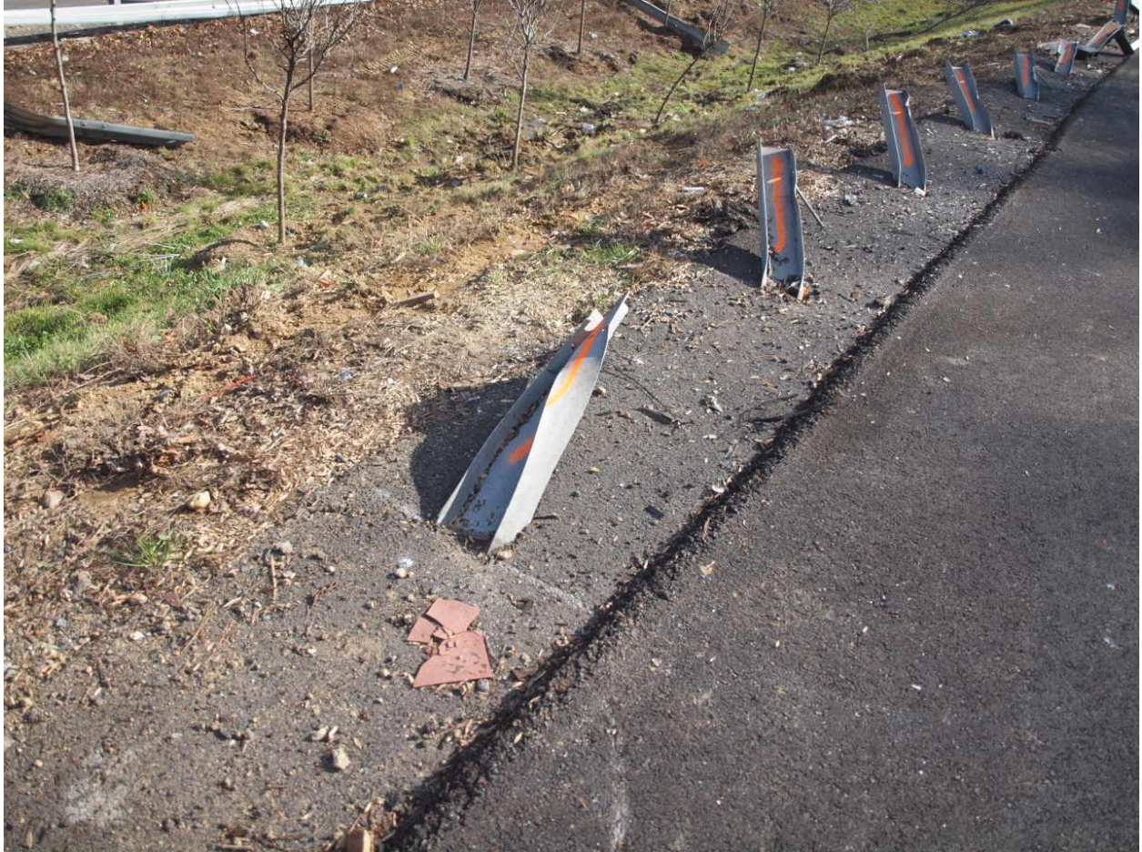
Highway Factors Photo 9 – Close up view of deformed W 6 x 9 steel I-beam posts standing in the paved shoulder adjacent to the leftmost travel lane in the eastbound direction looking to the southeast
