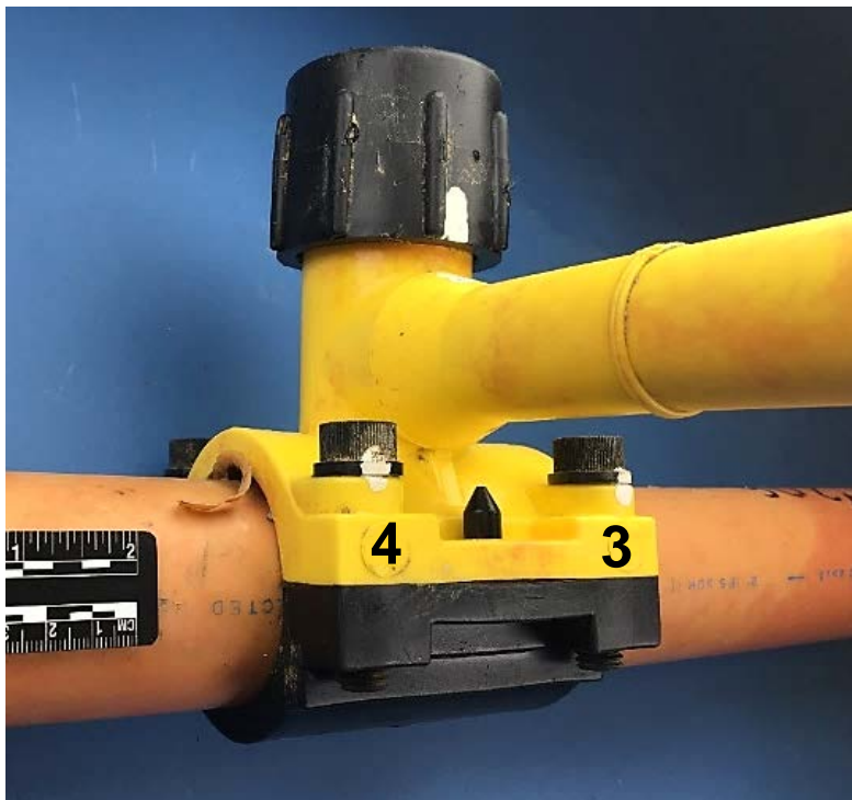
Figure 8. Photograph of the tee assembly from dwelling 206 showing intact bolts “3” and “4”.
