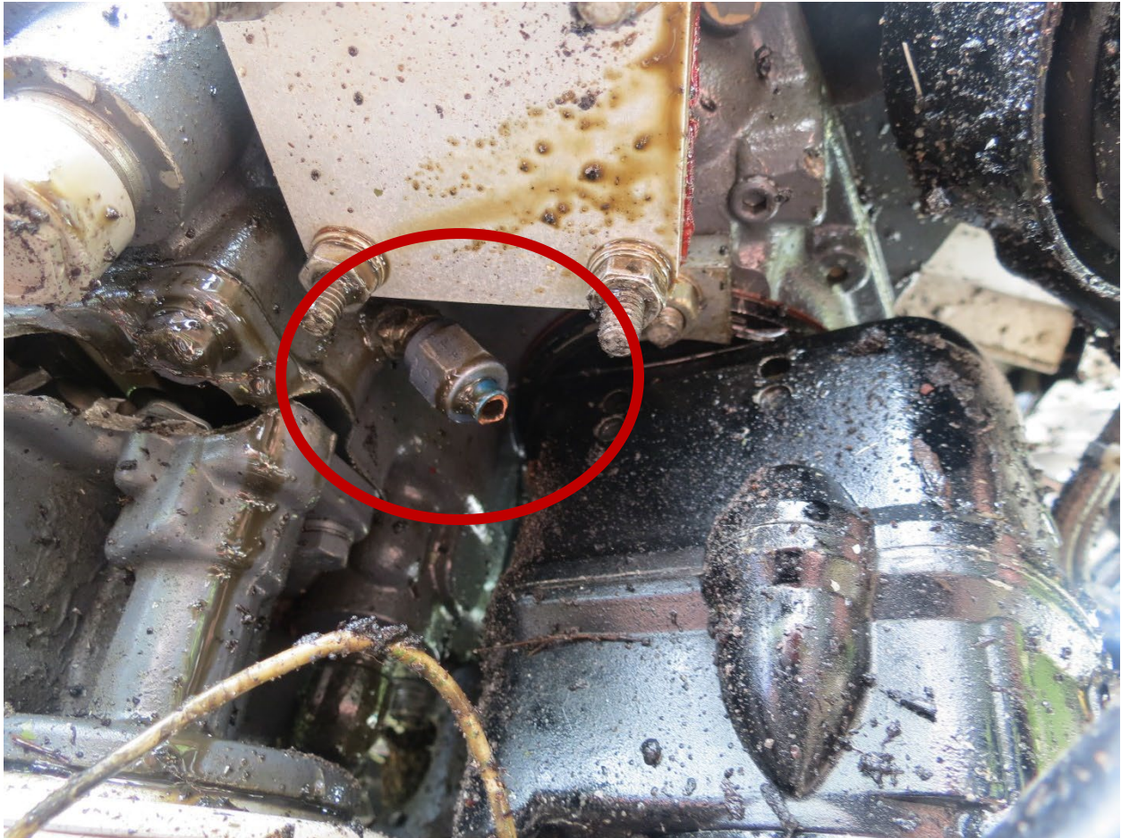
Figure 29. View of broken copper line installed on the accessory section of the engine.
