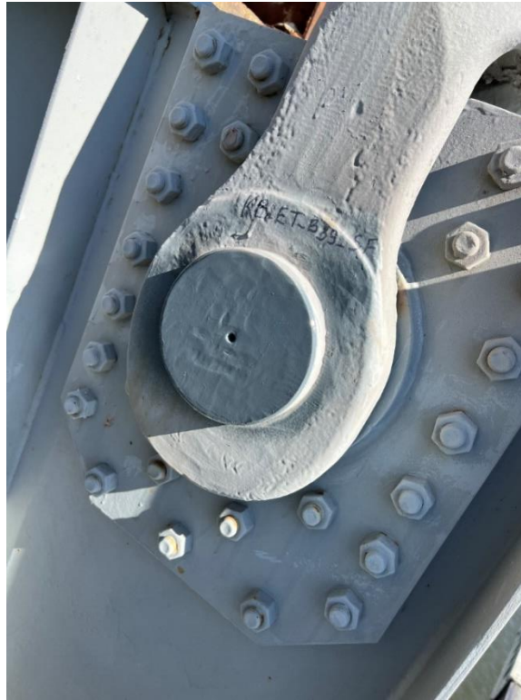
Figure 5: Pin face sprayed with cold galvanizing compound at Span 18, East Truss, B39, South Face (others similar)
