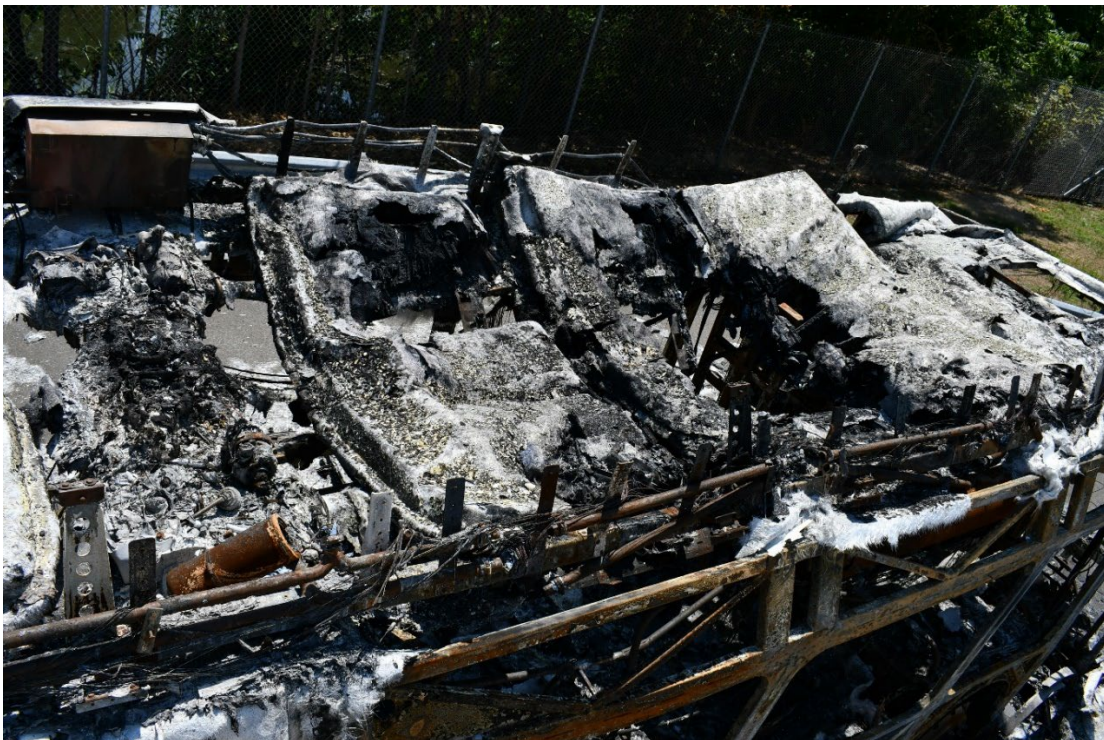
Figure 4: Post-fire rooftop energy storage enclosures
