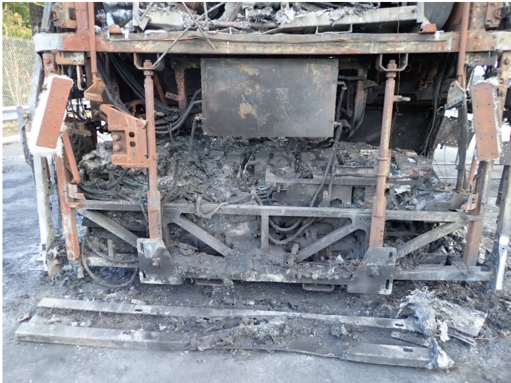
Figure 6: Post-fire rear mounted energy storage enclosures
