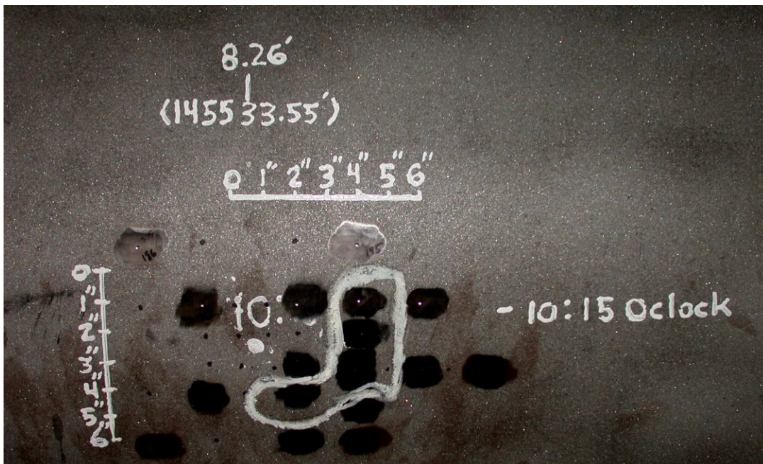
Figure 6. A view of hard spot region "A". The boundary of the hard spot indicates the region with hardness greater than 200 Brinell as determined by Telebrineller hardness testing.
