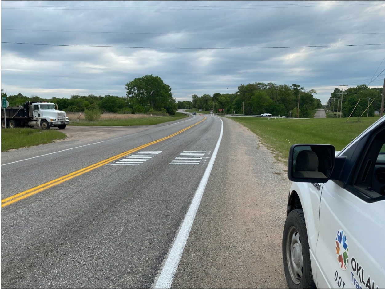
Figure 14. Close-up view of transverse rumble strips on eastbound SH 22 on the approach to the STOP sign. (source: ODOT)
