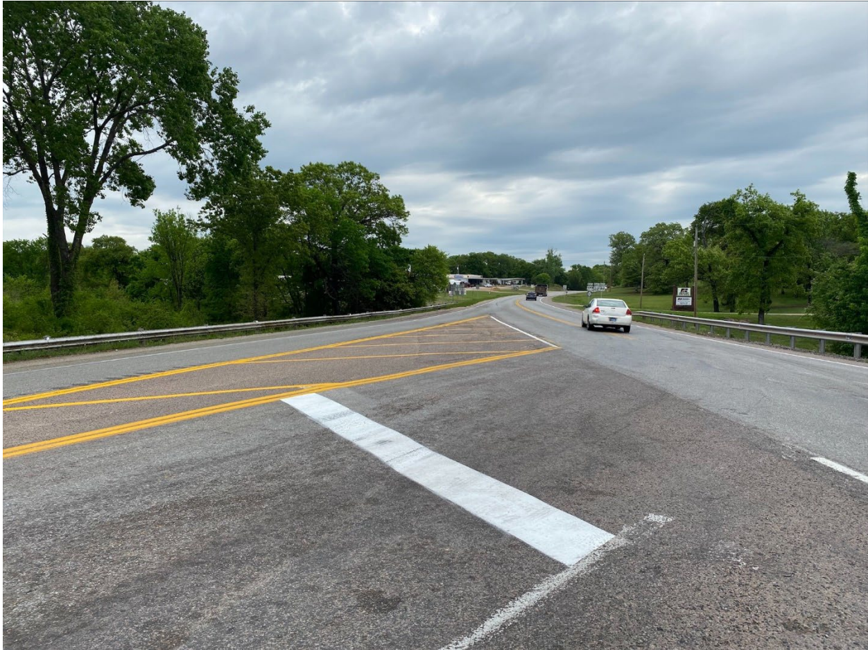
Figure 17. View of re-stripped STOP bar on eastbound SH 22. (source: Oklahoma DOT)
