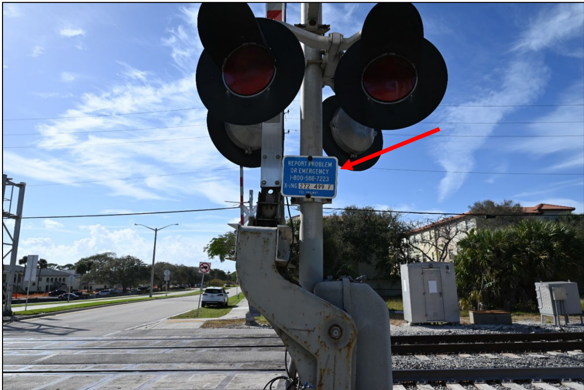
Figure 7: Westbound Hidden Valley Boulevard Emergency Signage
