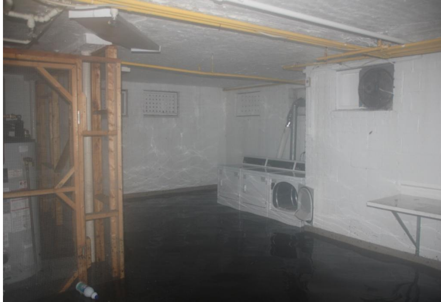
Figure 19: Photo of meter room in 8703 Arliss Street; Protective cage around water heater
