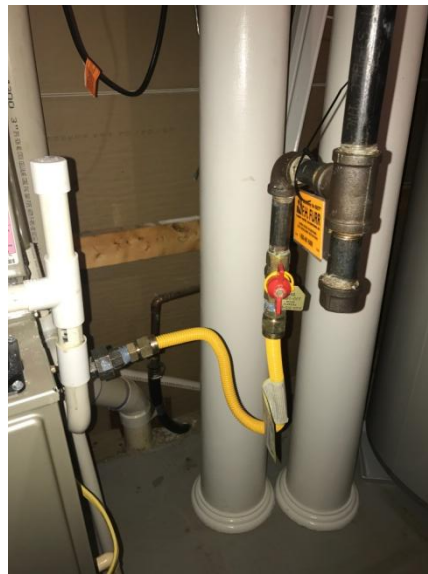
Photo showing use of flex connector/pig tail between steel house piping and appliance connection
