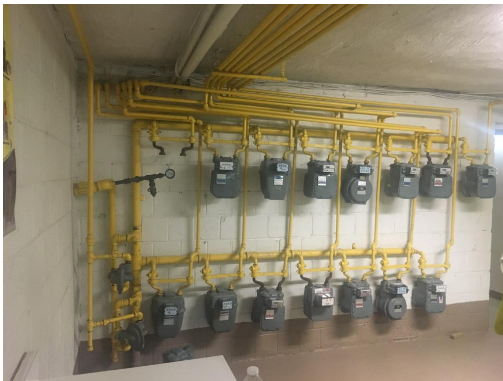
Figure 1: Exemplar meter and regulator assembly; located in Flower Branch Apartment complex
