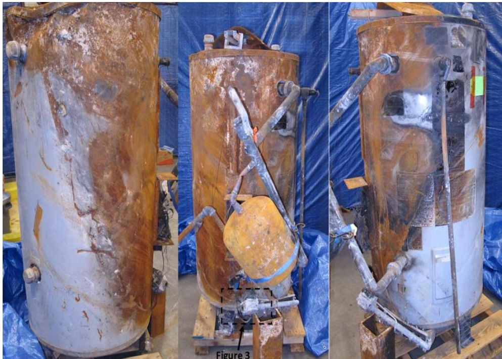
Figure 17: Water heater burn pattern
