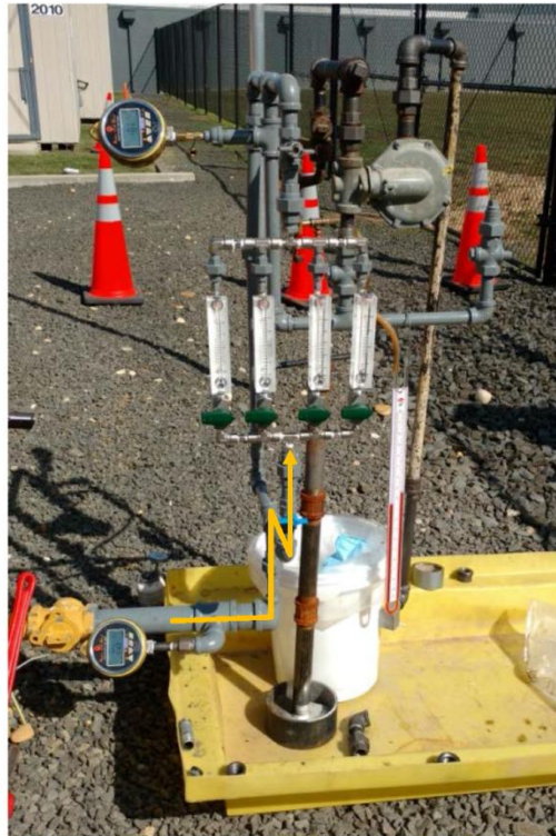
Figure 4. Mercury Regulator Test Apparatus, View 2 – Gas Path, Shown Using Yellow Arrow, is Directed towards the Rotameters, as Used during Relief Valve Flow Testing
