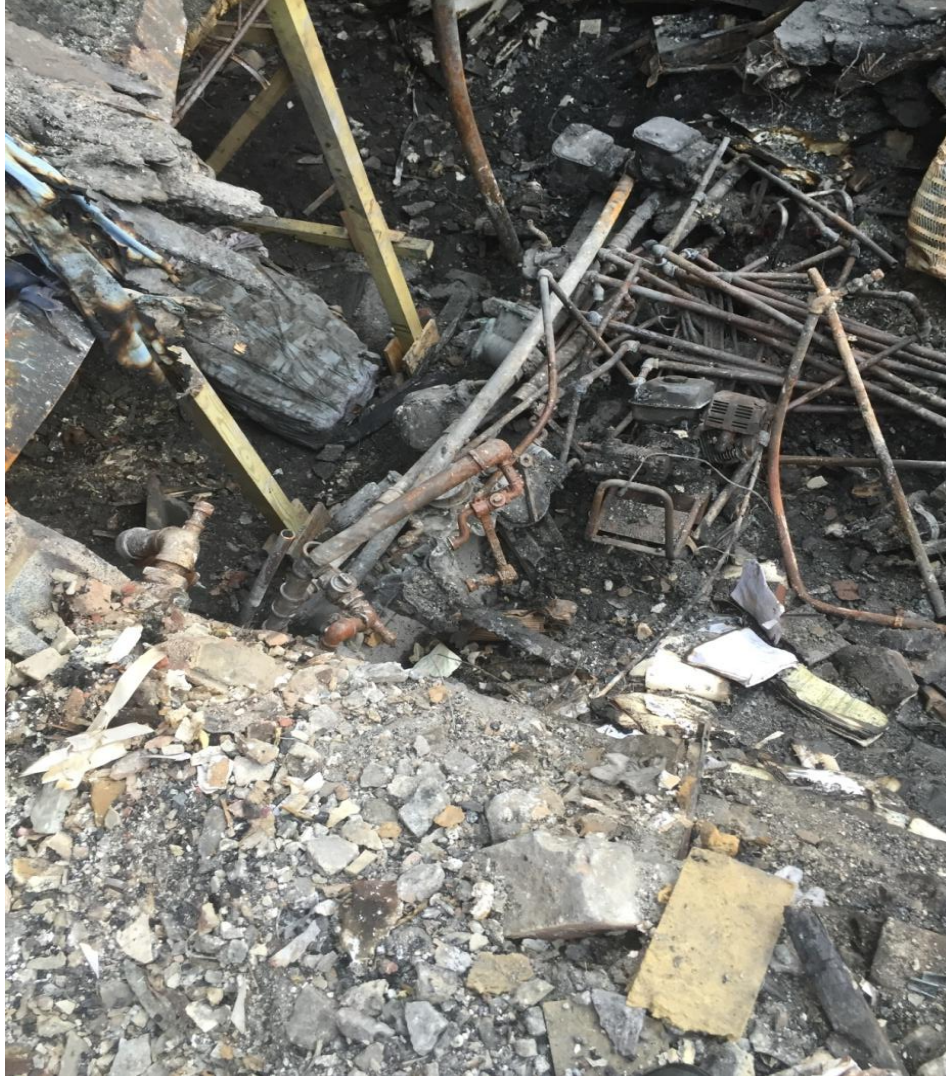
Figure 2: View into basement level meter/storage room of 8701 Arliss Street from grade level post removal of debris
