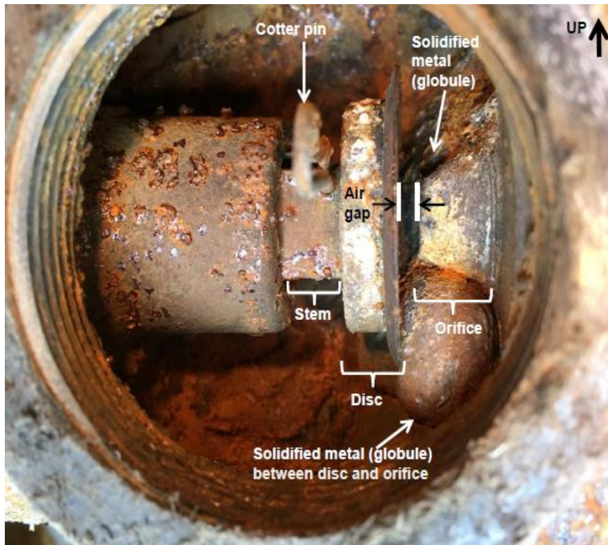
Figure 12: Lower gas regulator valve seat area
