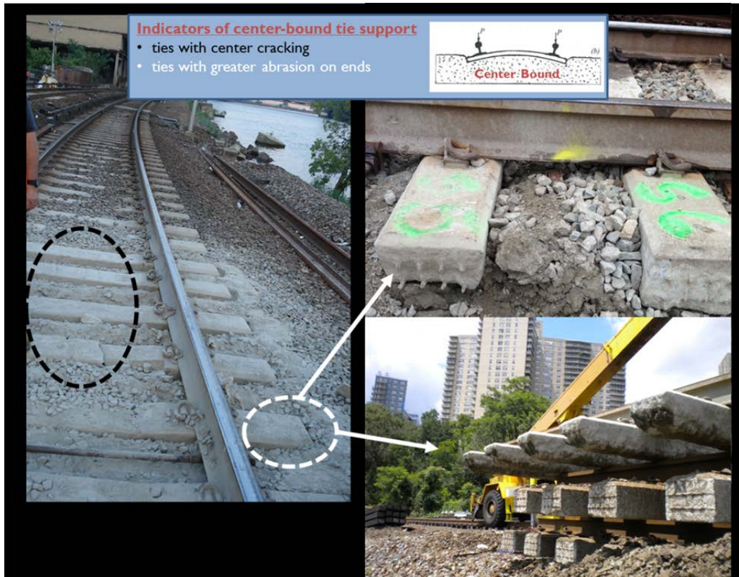
Figure 13: Indicators of center supported crossties (center-bound crossties).
