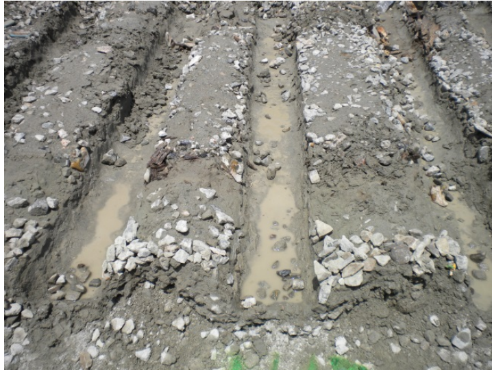
Figure 11: Presences of water beneath crossties and ballast layer.
