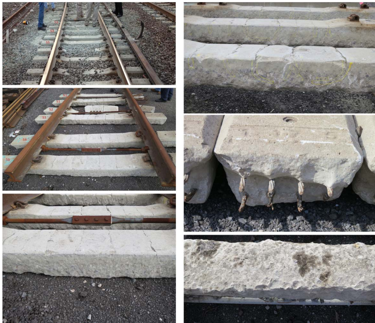
Figure 19: Concrete crossties in derailment curve: (19a, upper left) POD looking northbound – S2 broken; (19b, middle left) crossties near POD after removal – N1, S1, and S2 broken; (19c, lower left) close-up of crossties near POD after removal – reduced section of crossties; (19d, upper right) characterization of center cracks on crossties near POD; (19e, middle right) ends of crossties near POD; and, (19f, bottom right) typical bottom of crossties near POD.
