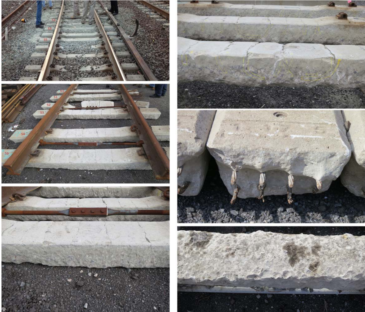
Figure 12: Damaged concrete cross-ties in derailment curve: (12a, upper left) POD looking northbound – S2 broken; (12b, middle left) cross-ties at POD after removal – N1, S1, and S2 broken; (12c, lower left) close-up of cross-ties at POD after removal – reduced section of cross-ties; (12d, upper right) characterization of center cracks on cross-ties near POD; (12e, middle right) ends of cross-ties near POD; and, (12f, bottom right) typical bottom of cross-ties near POD.
