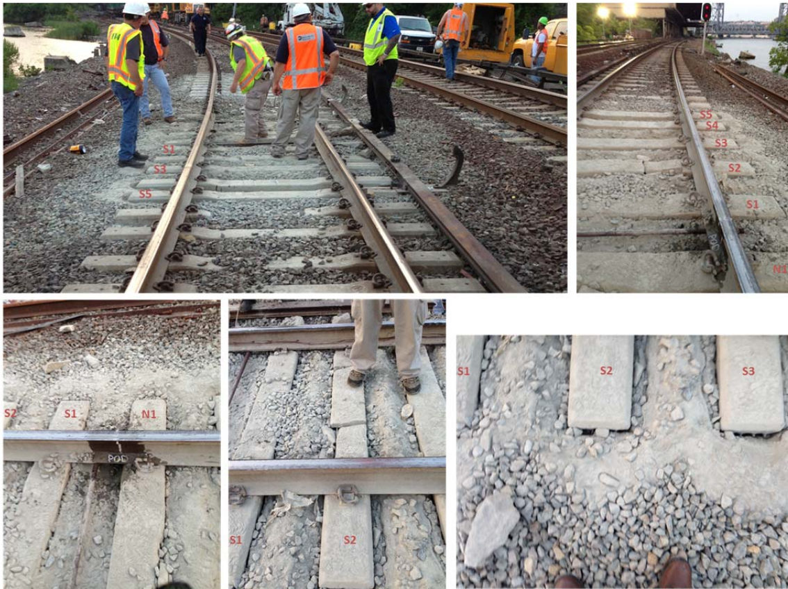
Figure 10: Damaged concrete crossties in derailment curve: (10a, upper left) POD looking northbound; (10b, upper right) POD looking southbound; (10c, lower left) POD facing gage side of inside rail; (10d, lower center) POD facing field side of inside rail; and, (10e, lower right) gaps at the crosstie-ends on inside of curve.
