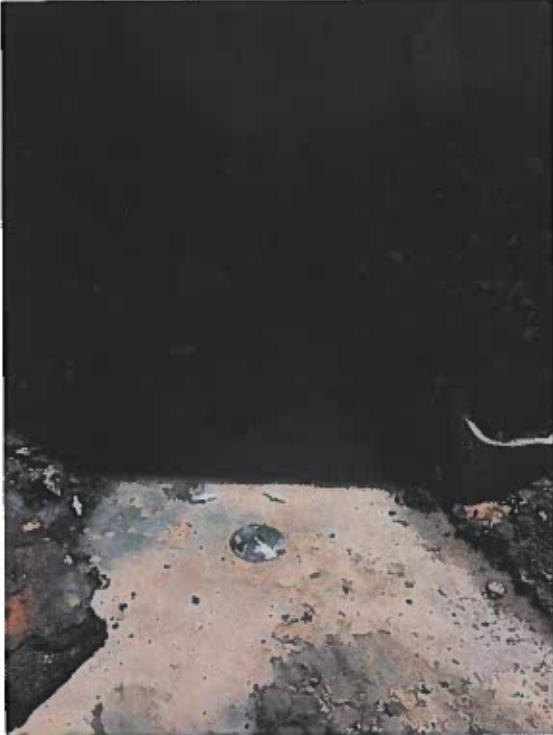
Vapor pin VP-06 installed near south wall.
