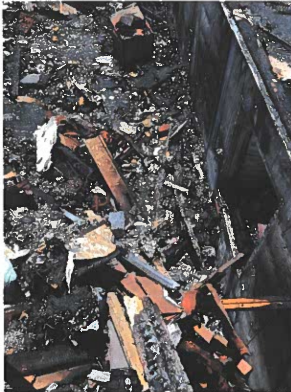
NW corner where vapor pin could not be installed due to debris.
